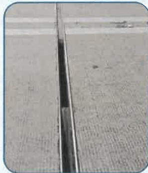
Figure 44: SRT WB Unsealed Bridge Deck Joints at Lake Vista Dr.
