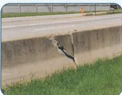
Figure 97: 360T SB Damaged Concrete Barrier South of SE Green Oaks Blvd.
