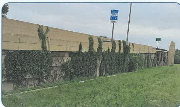
Figure 56: CTP SB MSE Wall Vegetation Overgrowth North of Clearfork Main St.
