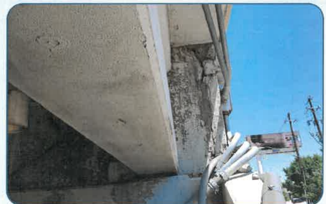
Figure 14: DNT Abutment Backwall Spall at Alpha Rd.
