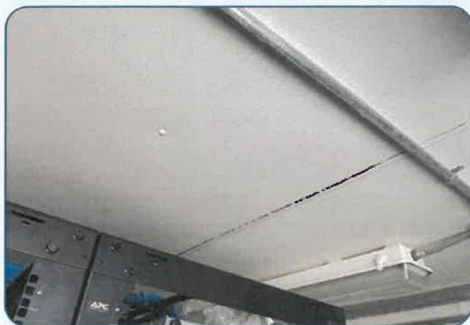
Figure 104: 360T MLG14 Fiber Hut Damaged Ceiling.
