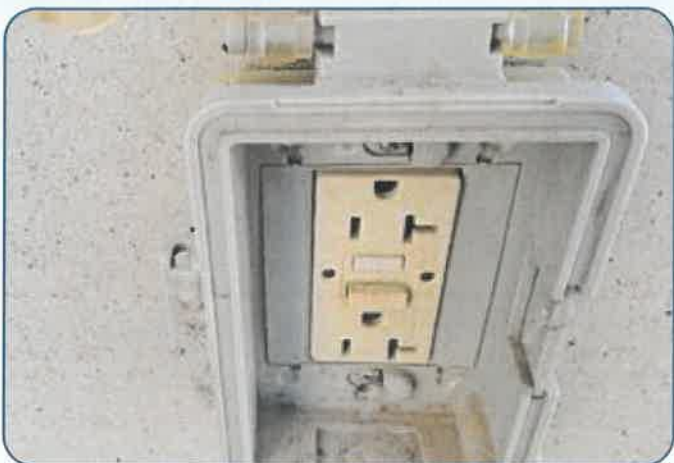
Figure 106: 360T MLG14 Failed Electrical Receptacle.
