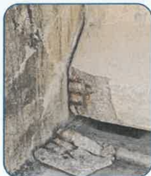
Figure 46: SRT EB Bridge Beam Spalling with Exposed Reinforcement East of N. MacArthur Blvd.
