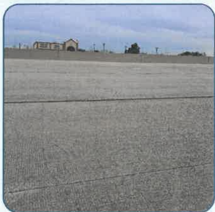
Figure 20: PGBT WB Unsealed Longitudinal Joint at IH-35E.
