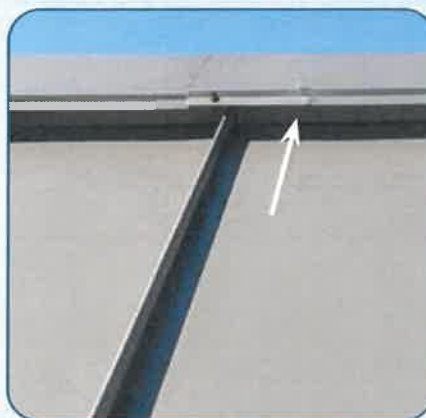
Figure 109: POC Damaged Roof.
