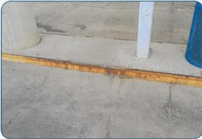
Figure 114: FOC Fuel Island Corrosion.
