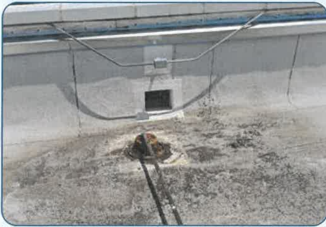
Figure 118: GE 5900 Deteriorated Roof.
