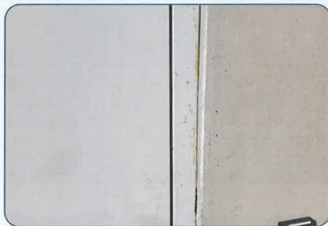
Figure 105: 360T MLG14 Fiber Hut Degraded Door Frame.
