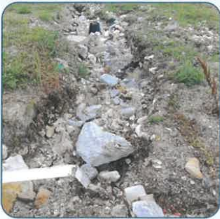
Figure 52: CTP NB Turf Erosion South of Dutch Branch Rd.
