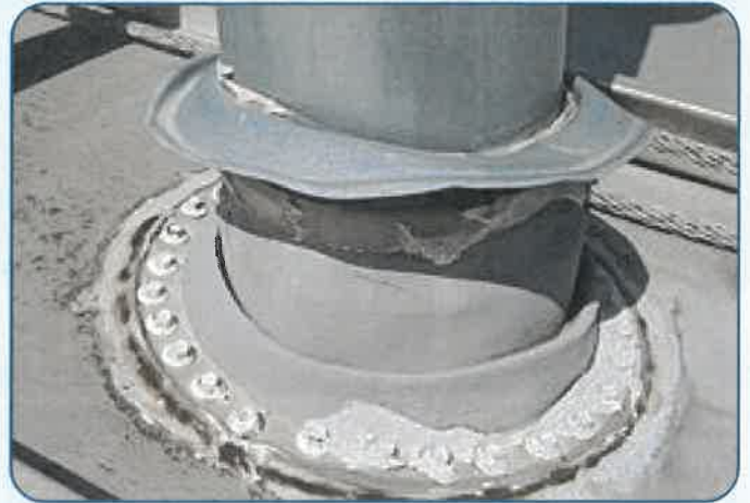
Figure 115: FOC Roof Failed Rain Hood.
