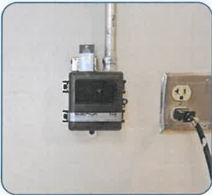
Figure 15: DNT MLP3 Non-Functioning CO Sensor.
