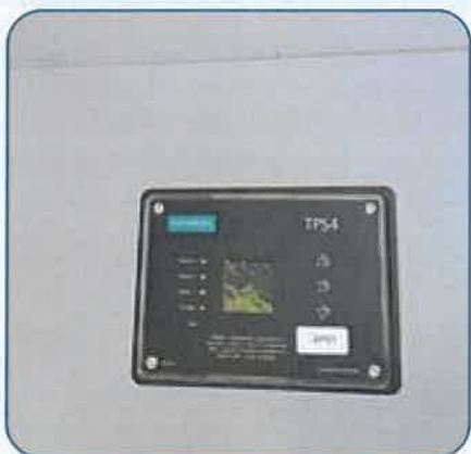
Figure 108: POC Switchboard SESB Alarmed Surge Suppressor.
