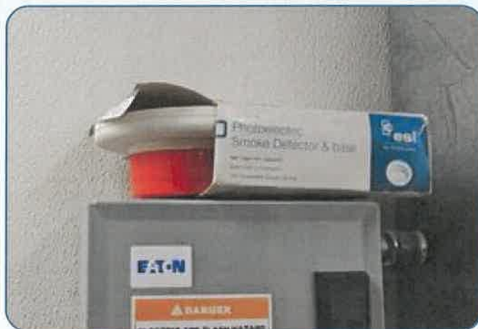
Figure 64: CTP MLG3 Non-Installed Smoke Detector.
