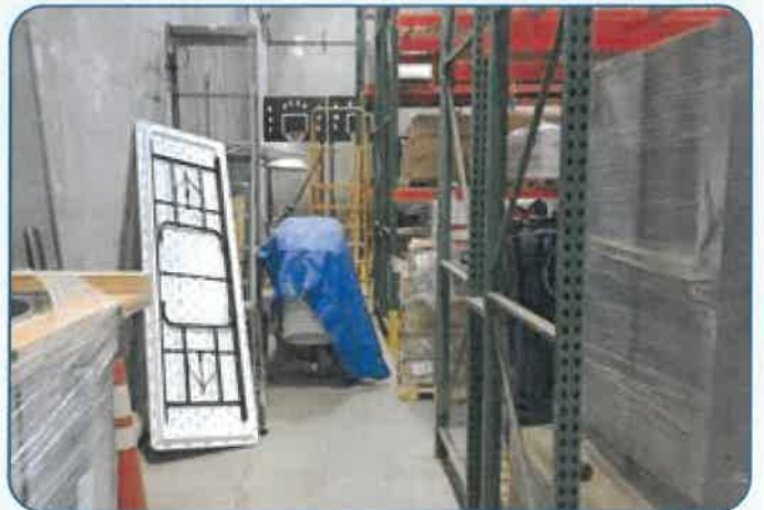
Figure 117: FOC Warehouse Blocked Egress Route.
