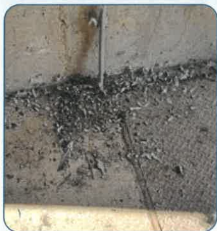
Figure 82: LLTB Electrical Room Bird-Insect Infestation.
