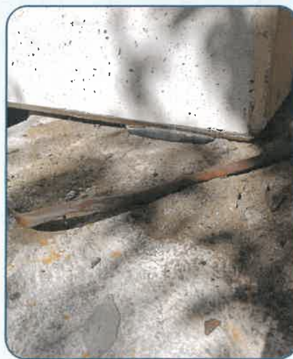
Figure 102: 360T Bridge Deformed Bearing Pad SB Frontage Road Over Fish Creek.
