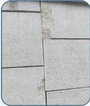
Figure 41: SRT WB MSE Wall Panel Racking and Spalling at Ohio Dr.
