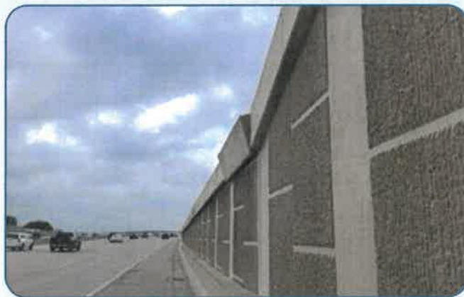
Figure 25: PGBT WB Wall Coping Displacement at Old Denton Rd.
