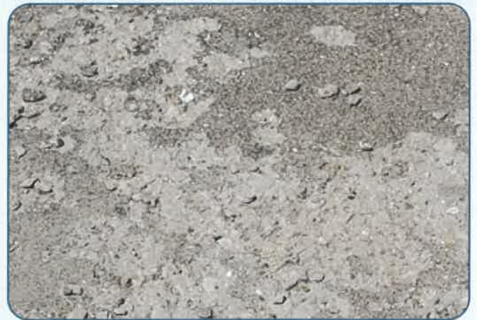
Figure 63: CTP MLG3 Deteriorated Landing.
