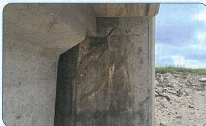
Figure 61: CTP SB Bridge Backwall Spalling North of CR 1016.
