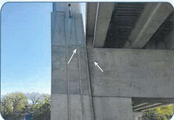
Figure 78: LLTB Minor Cap Column Cracking at the East End.
