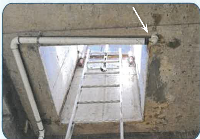
Figure 80: LLTB Electrical Room Separated Drain Pipe.
