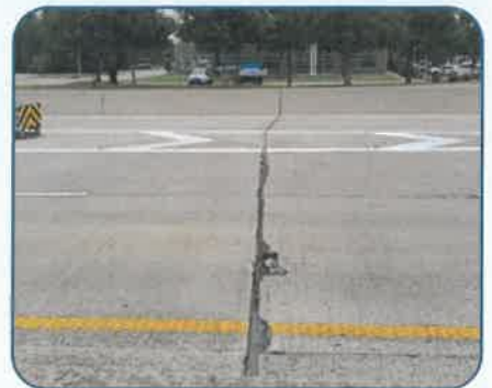
Figure 7: DNT NB Pavement Spalling North of Plano Pkwy.
