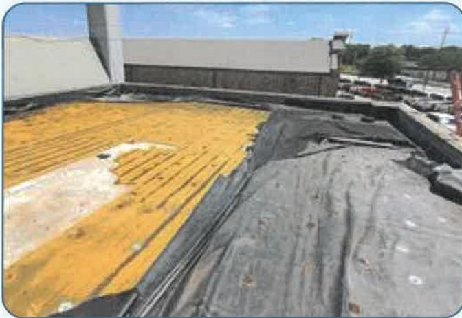
Figure 91: AATT Gantry Deteriorated Roof.
