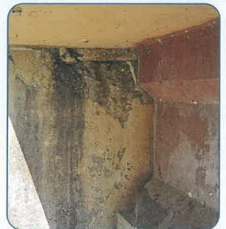
Figure 71: MCLB Abutment Backwall Cracking and Spalling.
