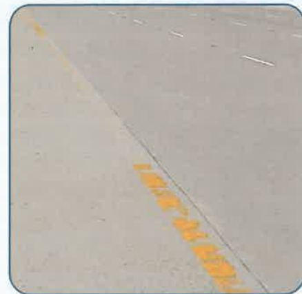
Figure 38: SRT WB Damaged or Faded Pavement Markings West of Coit Rd.
