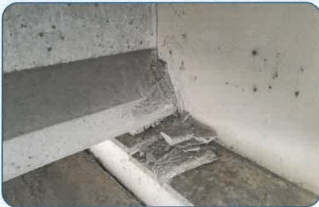
Figure 27: PGBT Concrete Beam Spall at Royal Ln.
