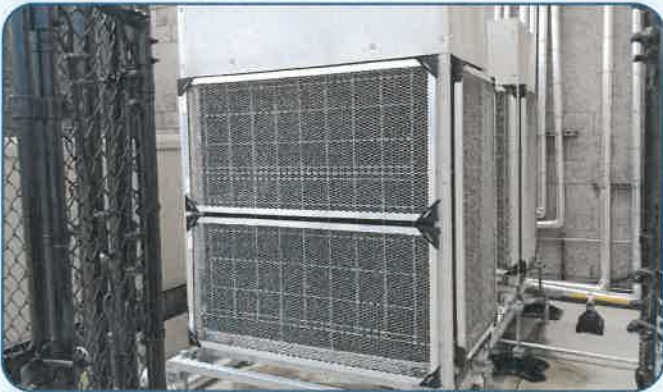
Figure 137: MLP 6 – HVAC Replacement.
