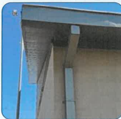
Figure 112: POC Damaged Gutter.
