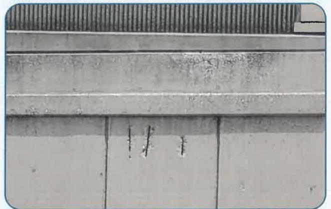
Figure 9: DNT NB MSE Wall Spalling with Exposed Reinforcement North of Cedar Springs Rd.
