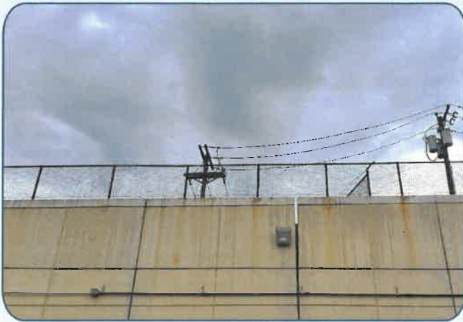
Figure 89: AATT Cracking, Spalling and Stained Wall Panels at West Side.
