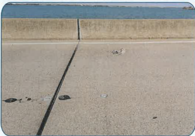
Figure 67: MCLB Deck Spalling.
