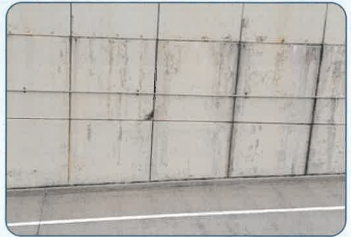
Figure 90: AATT Cracking, Spalling and Stained Wall Panels at East Side.
