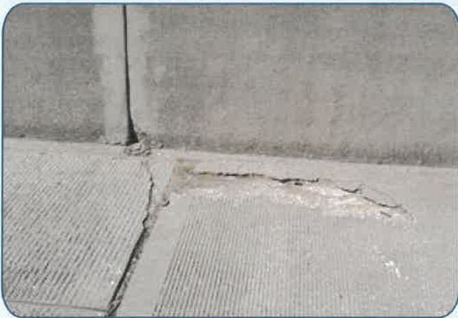
Figure 76: LLTB Approach Slab Spalling.
