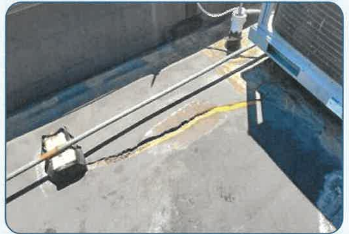
Figure 92: AATT Gantry Electrical Room Damaged Roof.
