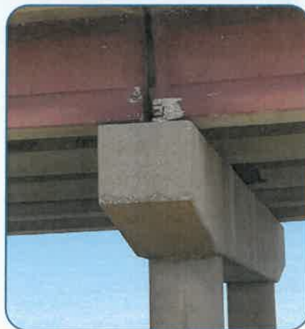
Figure 70: MCLB Concrete Bridge Beam Spalling with Exposed Reinforcement.
