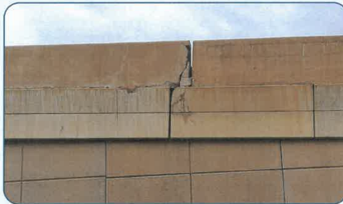
Figure 55: CTP NB MSE Wall Rail and Coping Cracking North of SH 183.
