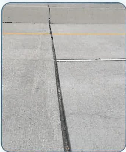
Figure 101: 360T Bridge Relief Joint with Debris North of N. Holland Rd.
