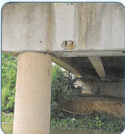
Figure 69: MCLB Bent Cap Spalling with Exposed Reinforcement.
