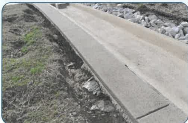
Figure 23: PGBT NB Turf Erosion and Flume Undermining South of Telecom Pkwy.
