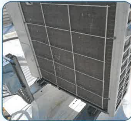
Figure 16: DNT MLP4 Roof HVAC Unit without Hail Guard.
