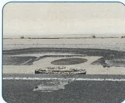
Figure 6: DNT NB Inlet Damage North of Lemmon Ave.
