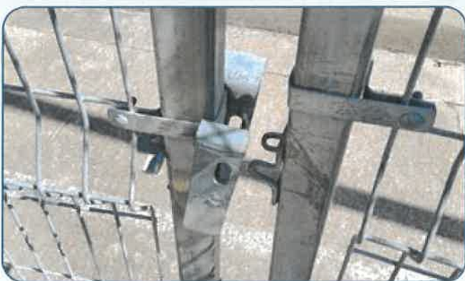
Figure 18: DNT Fiber Hut 1 Uncloseable Gate Lock.
