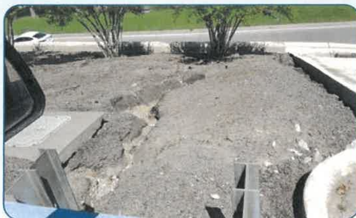
Figure 24: PGBT WB Landscape Bed Erosion at Coit Rd.
