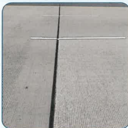
Figure 58: CTP NB Unsealed Bridge Joint at S. Hulen St.
