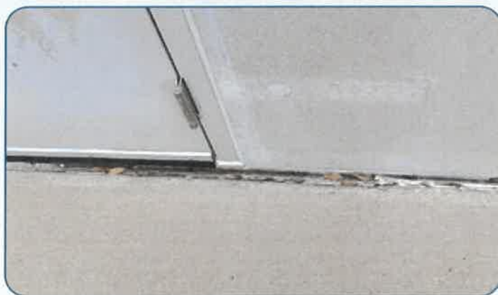
Figure 73: MCLB Fiber Hut Exterior Joint Failure.
