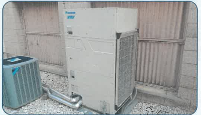
Figure 138: MLP 8 – HVAC Upgrade.
