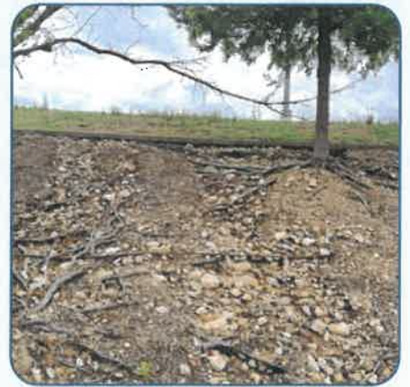
Figure 54: CTP SB Landscape Bed Erosion South of Overton Ridge Blvd.
