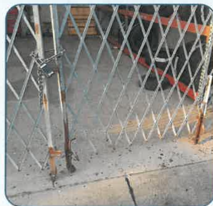
Figure 113: POC Storage Building Corroded Gate.
