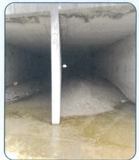
Figure 103: 360T Bridge Class Culvert with Sediment Buildup North of Webb Lynn Rd.
