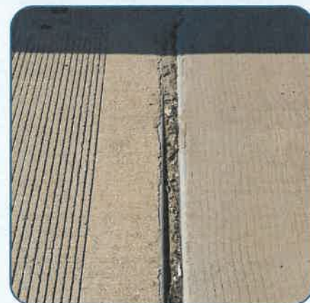
Figure 59: CTP SB Debris Filled Relief Bridge Joint at W Risinger Rd.
