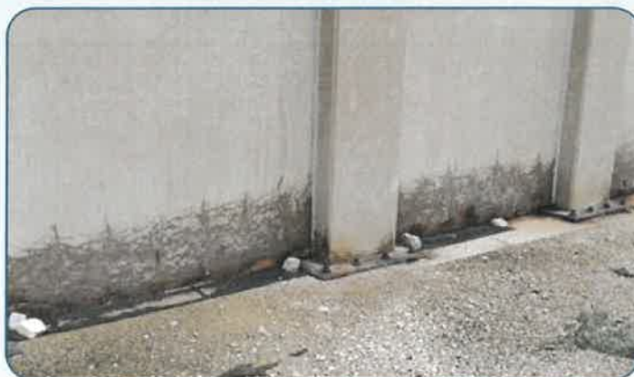
Figure 48: SRT IH-35E Winter Weather Operations Facility Degraded Wall.
