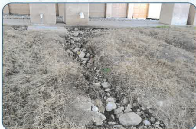
Figure 60: CTP SB Bridge Column Drainage System Erosion at IH-20.
