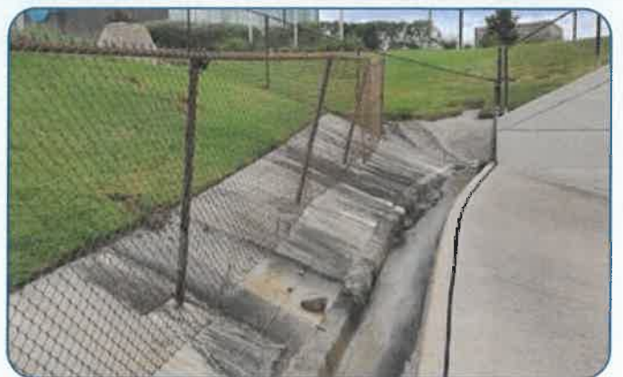
Figure 88: AATT Fence Damage.
