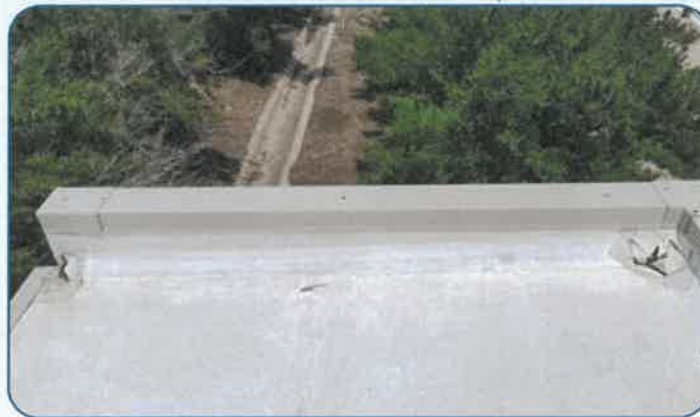
Figure 47: SRT MLG1 Fiber Hut Damaged Roof.
