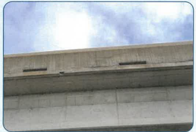
Figure 77: LLTB Deck Overhang Spalling.
