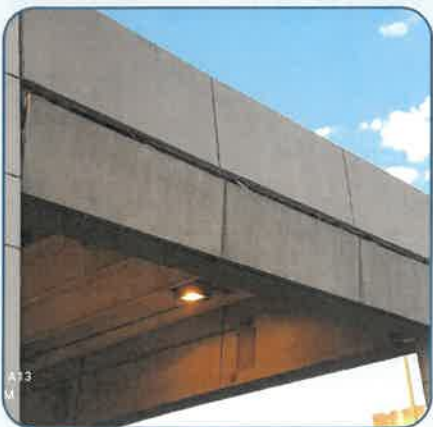
Figure 33: PGBT Midway On-Ramp Gantry Separated Wall Panel 2.
