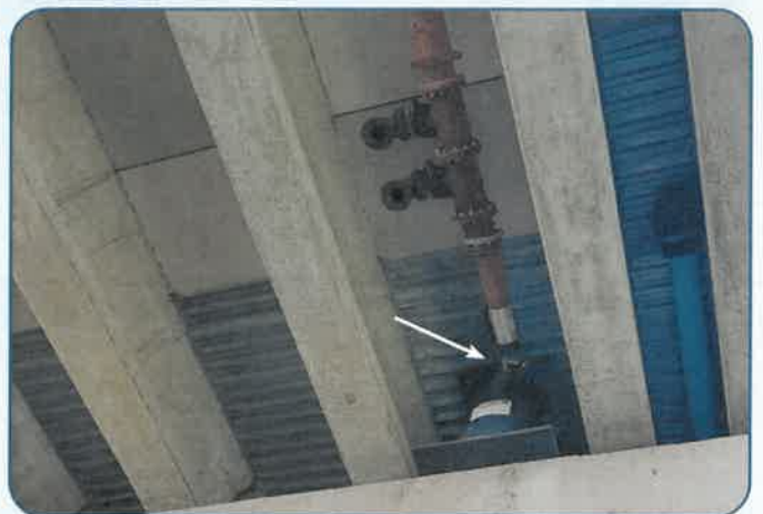
Figure 79: LLTB Damaged Pipe of Bridge Collection Runoff System.
