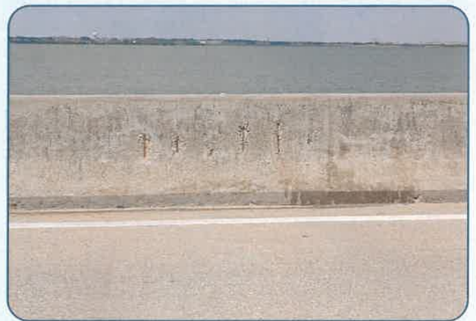
Figure 68: MCLB Concrete Rail Spalling with Exposed Reinforcement.
