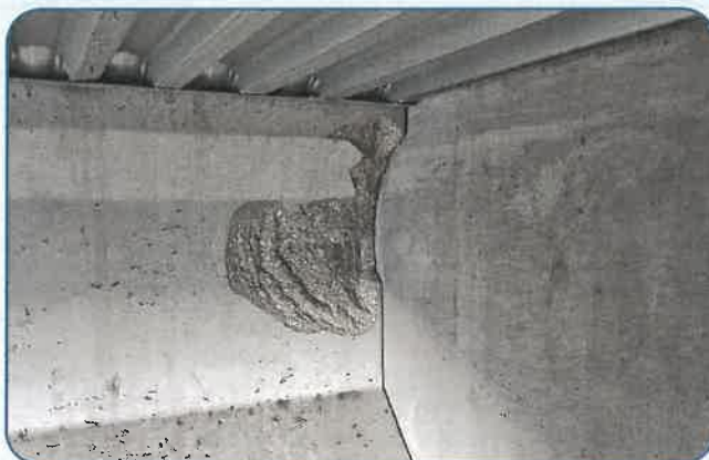
Figure 13: DNT Bridge Beam Spalling at Eldorado Pkwy.
