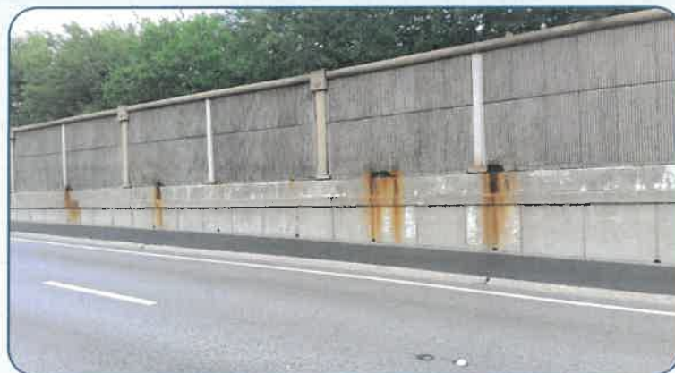
Figure 10: DNT SB Wall Staining South of Glenwick Ln.
