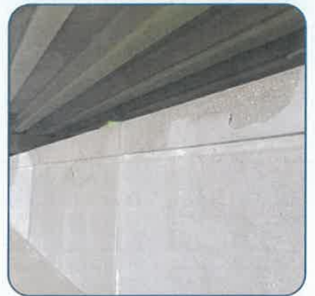
Figure 35: PGBT Oakdale Road Winter Weather Operations Facility Damaged Wall.
