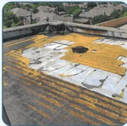
Figure 31: PGBT Eastbound Renner Road On-Ramp Deteriorated Roof.
