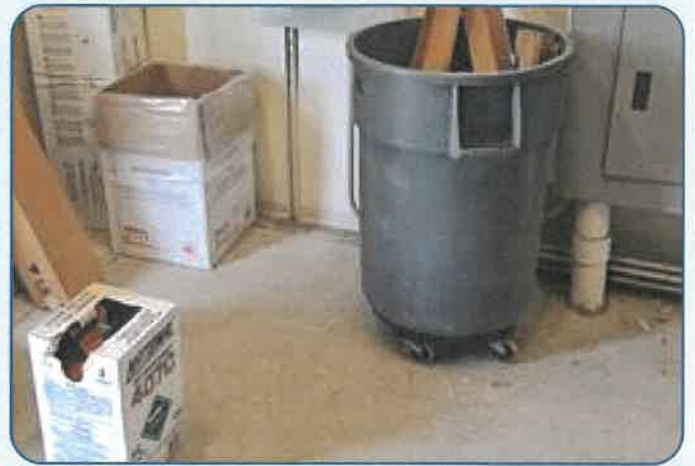
Figure 119: GE 5910 Electrical Room Improper Storage.
