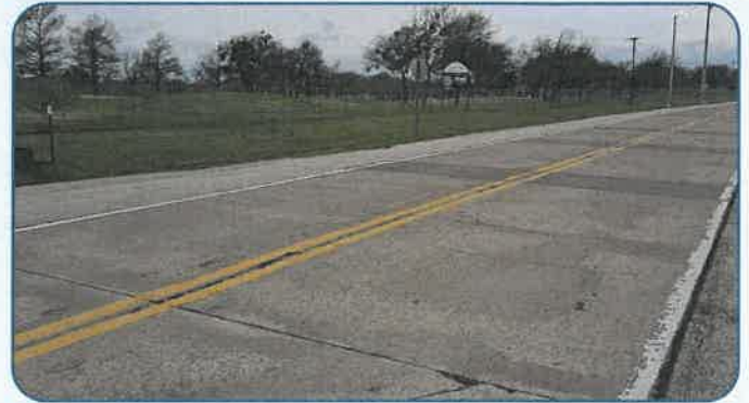
Figure 66: MCLB EB Damaged or Faded Pavement Markings at West Approach.
