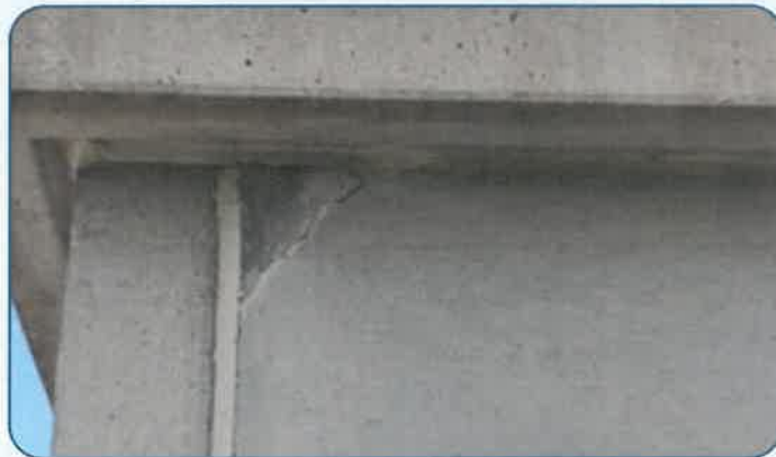
Figure 72: MCLB Fiber Hut Exterior Wear and Crack.
