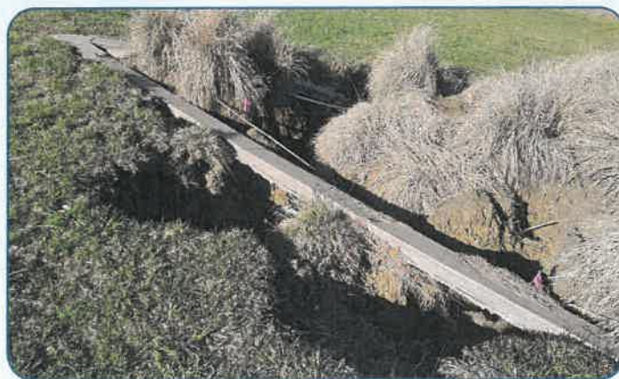
Figure 40: SRT WB Landscape Bed Concrete Edging Undermining West of W. Hebron Pkwy.
