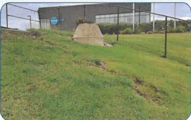
Figure 87: AATT Turf Erosion at East End.
