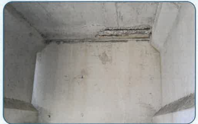
Figure 12: DNT Underdeck Spall with Exposed Reinforcement at IH 635.
