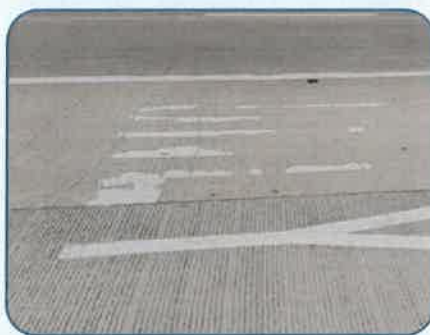
Figure 99: 360T Damaged or Faded Pavement Markings at US 287.
