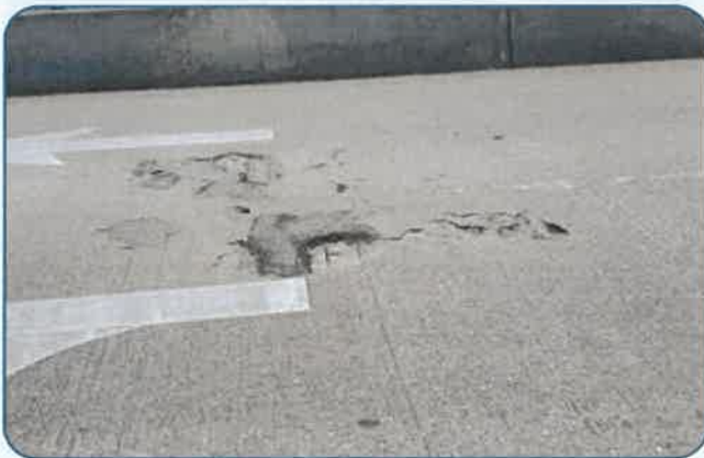
Figure 11: DNT Deck Spalling at IH 635.
