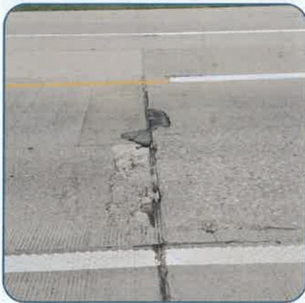
Figure 49: CTP NB Pavement Punchout North of McPherson Blvd.
