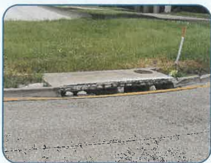
Figure 98: 360T SB Curb Inlet Damage with Exposed Reinforcement at SE Green Oaks Blvd.
