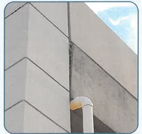
Figure 32: PGBT Midway On-Ramp Gantry Separated Wall Panel 1.
