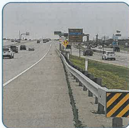
Figure 37: SRT EB Unsealed Longitudinal Shoulder Pavement Joint East of N. Josey Ln.
