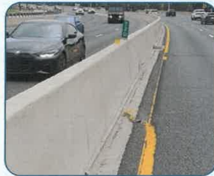
Figure 4: DNT SB Damaged or Faded Pavement Markings South of Sojourn Dr.
