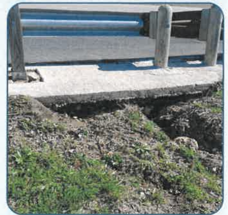
Figure 51: CTP SB MBGF Mow Strip Undermining North of Dutch Branch Rd.
