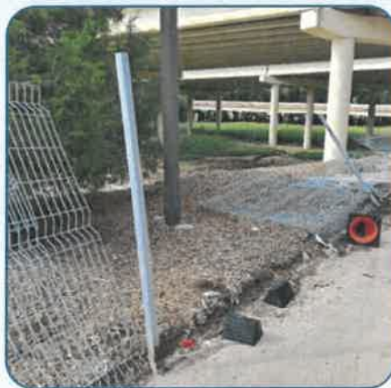
Figure 34: PGBT Brand Road Winter Weather Operations Facility Damaged Fence.
