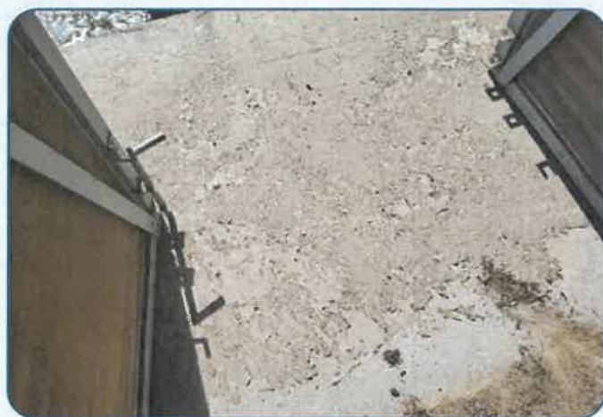
Figure 81: LLTB Damaged Concrete Landing.
