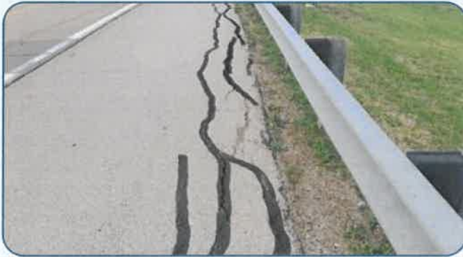
Figure 65: MCLB WB Asphalt Shoulder Cracking.
