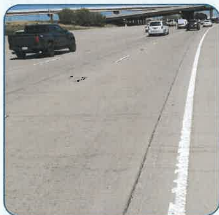
Figure 36: SRT EB Unsealed Longitudinal Pavement Joint West of Old Denton Rd.
