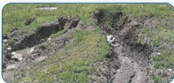
Figure 100: 360T NB Turf Erosion North of Heritage Pkwy.
