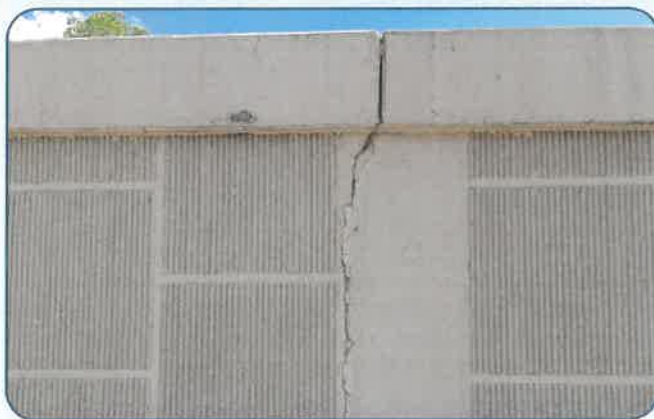
Figure 26: PGBT EB Wall Cracking West of Independence Pkwy.
