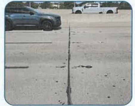
Figure 3: DNT NB Unsealed Pavement Joints South of W. Park Blvd.
