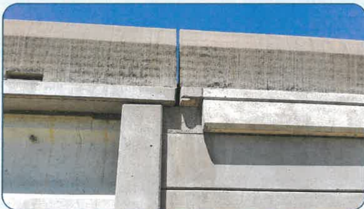
Figure 75: LLTB MSE Wall Coping Damage.
