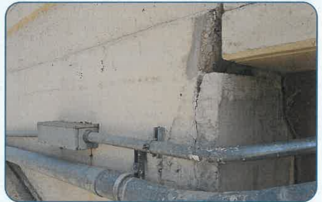
Figure 28: PGBT Backwall Cracking and Spalling at Gateway Dr.
