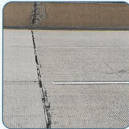
Figure 50: CTP SB Pavement Joint Deterioration and Barrier Spall South of Arborlawn Dr.
