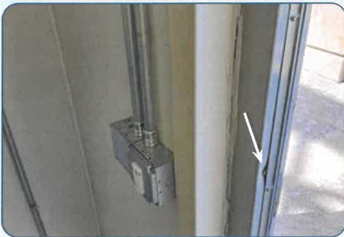
Figure 62: CTP MLG1 Fiber Hut Deteriorated Seal.
