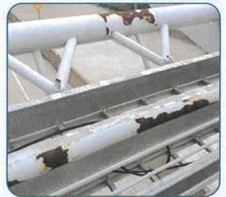
Figure 17: DNT MLP4 Gantry Coating Failure.
