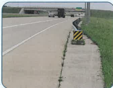
Figure 95: 360T NB Unsealed Longitudinal Joint South of Ragland Rd.
