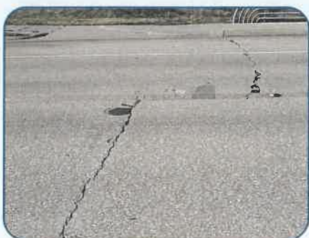
Figure 96: 360T SB Pavement Cracking South of Lone Star Rd.
