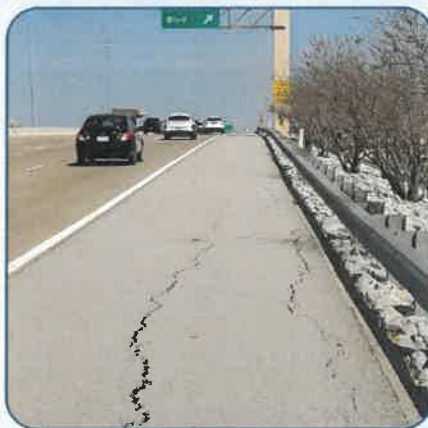
Figure 21: PGBT EB Asphalt Shoulder Cracking West of SH 114.
