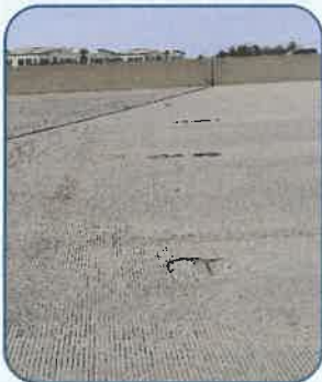
Figure 43: SRT EB Bridge Deck Spalling at Coit Rd.
