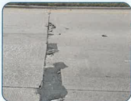
Figure 94: 360T NB Spalled Pavement Joint North of Doryn Dr.
