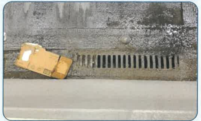
Figure 86: AATT Obstructed Grate Inlet within Tunnel.
