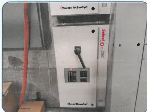
Figure 93: AATT Main Electrical Room Failed Surge Suppressor.
