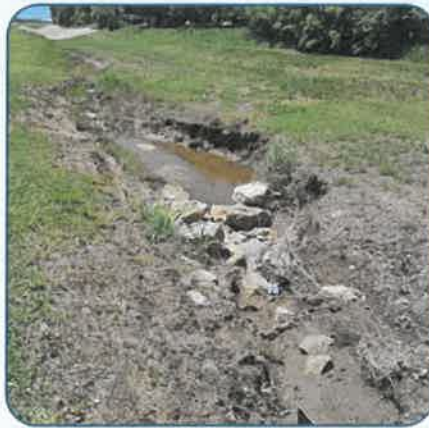
Figure 53: CTP SB Minor Ditch Erosion South of W FM 917.
