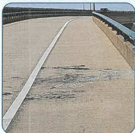
Figure 57: CTP SB Bridge Deck Spalling at CTP to IH 20 WB DC.
