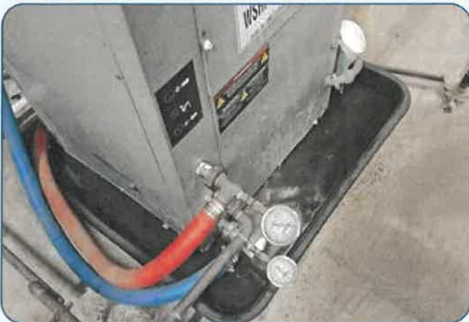
Figure 116: FOC HVAC Unit Leak.
