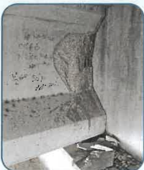
Figure 45: SRT WB Bridge Beam Spalling at Standridge Dr.
