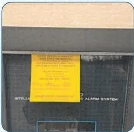
Figure 30: MLP7 Yellowed-Tagged Fire Alarm Control Panel.
