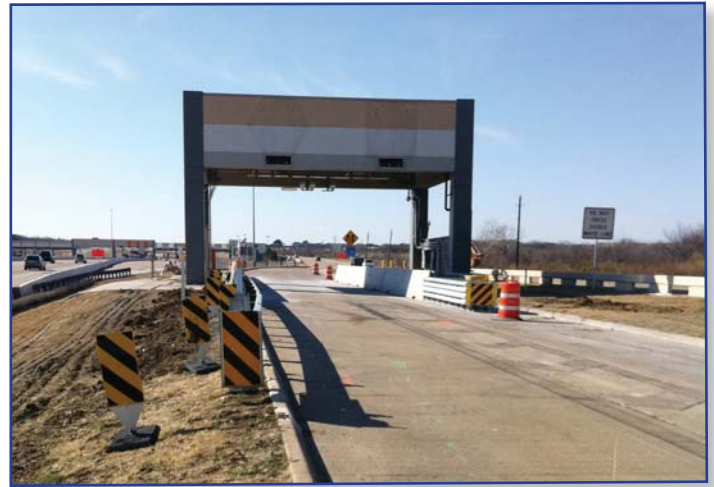
Southbound exit ramp from PGBT to Belt Line Road after concrete replacement for the All-ETC ramp modifications project.
