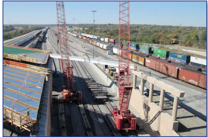
Crews erecting concrete beams for southbound CTP main lanes over the rail yard in Fort Worth.
