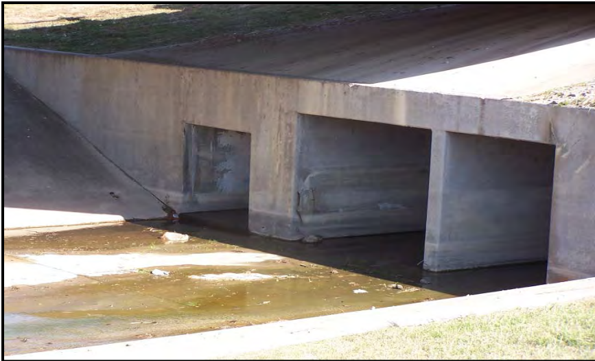
Photo 3. Water 4 – Looking southeast from north of SRT at stream as it exits culvert at edge of ROW.
