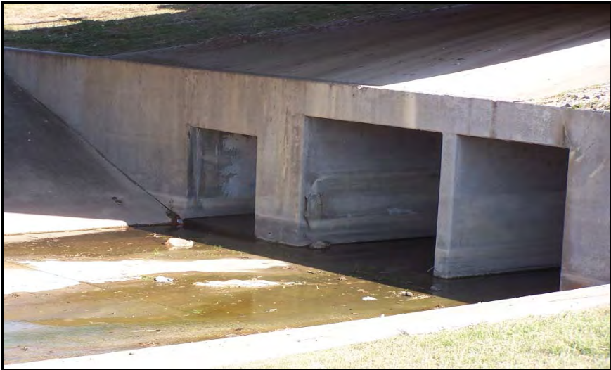
Photo 3. Water 4 – Looking southeast from north of SRT at stream as it exits culvert at edge of ROW.
