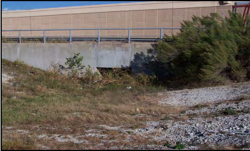
Photo 1. Water 1 – Looking east from west side of DNT culvert at edge of ROW.
