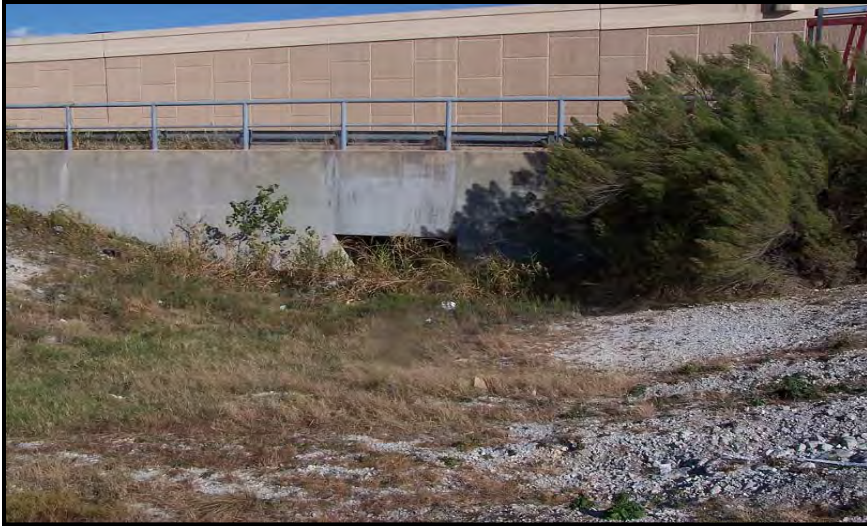
Photo 1. Water 1 – Looking east from west side of DNT culvert at edge of ROW.
