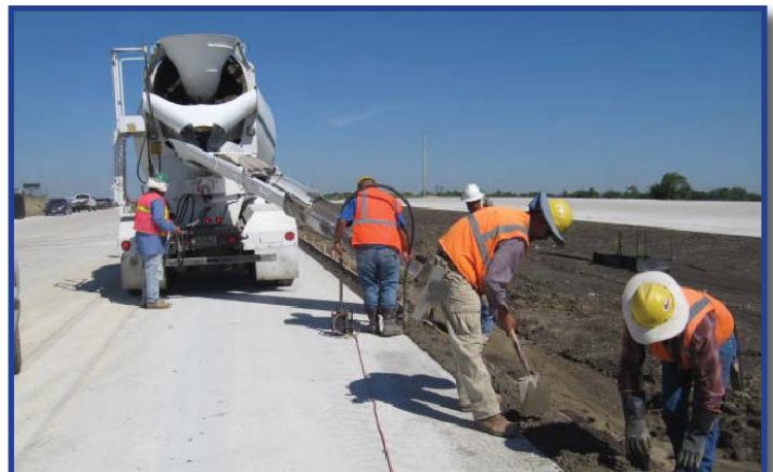
On the PGBT Eastern Extension project, crews pour concrete off the eastbound main lane north of Hickox Road in Section 29, which extends through Rowlett and Sachse.
