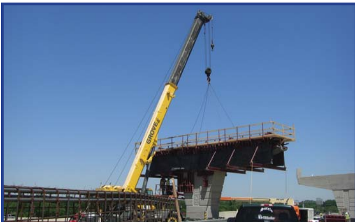
On the PGBT Western Extension project, crews set formwork for a bridge support at I-20 in Grand Prairie.
