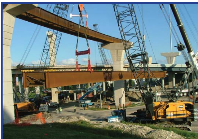
Crews use cranes to lift a massive steel bridge beam into place on the SRT/DNT interchange in Frisco and Plano.
