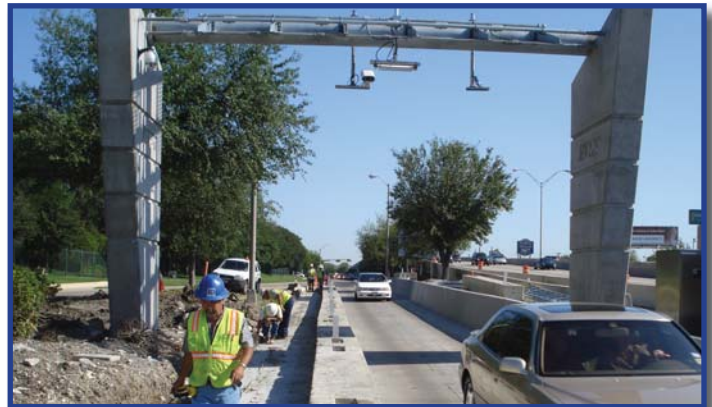
All-ETC work continued on the DNT with gantry construction at Keller Springs Road in far North Dallas.
