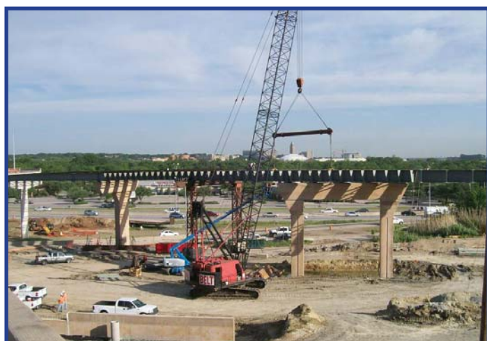
CTP crews set beams for the Rosedale Street connector bridges near I-30 in Fort Worth.
