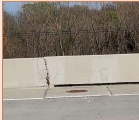
Figure 19: PGBT concrete rail cracking NBML between Miller Rd. and Main St.
