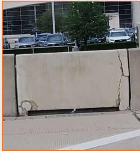
Figure 36: SRT concrete rail cracking and spalling SBML north of Leadership Dr.
