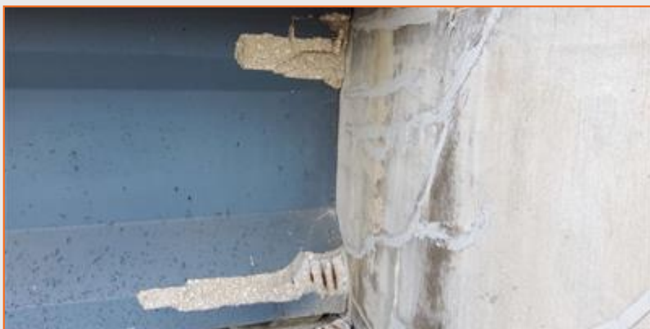
Figure 11: DNT bridge beam spalling with exposed reinforcement SBML at Eldorado Pkwy.
