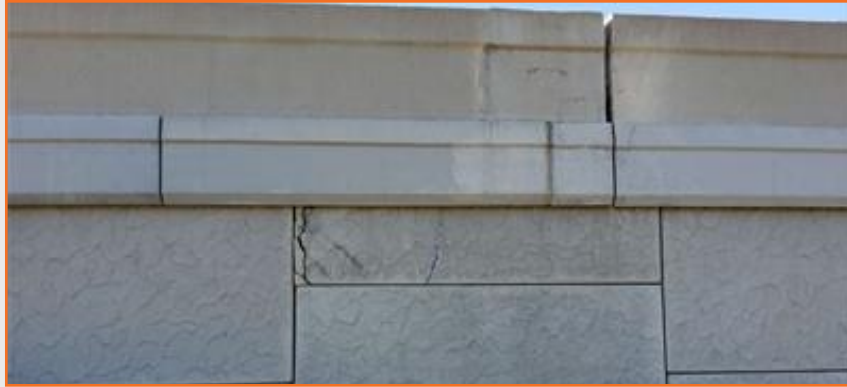
Figure 78: 360T MSE wall panel cracking and spalling NBML north of FM 2011.
