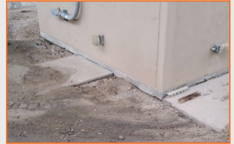
Figure 48: SRT Fiber Hut drainage concern and undermining of building.
