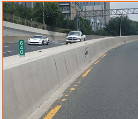
Figure 6: DNT pavement markings faded or missing NBML north of Arapaho Rd.
