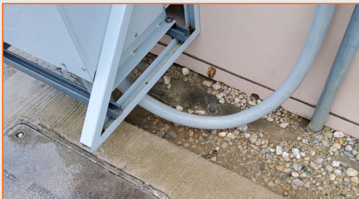
Figure 58: CTP Fiber Hut at FM 1187 runoff entering building.
