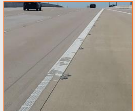
Figure 23: PGBT pavement markings faded or missing SBML north of Pioneer Pkwy.
