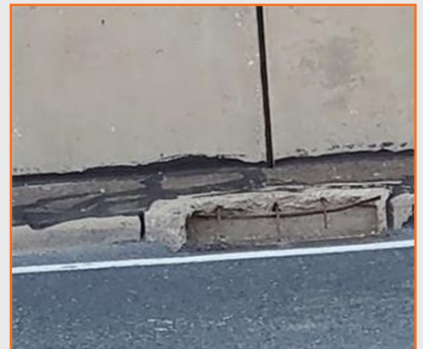
Figure 7: DNT curb inlet damage NBML south of Oak Lawn Ave.
