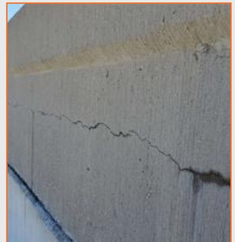
Figure 81: 360T bridge rail cracking NBML south of Heritage Pkwy.
