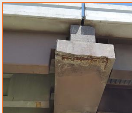
Figure 9: DNT bridge bent cap spalling with exposed reinforcement SBML at IH-635.
