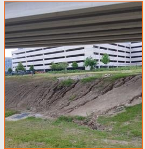
Figure 37: SRT embankment erosion NBML south of DNT.
