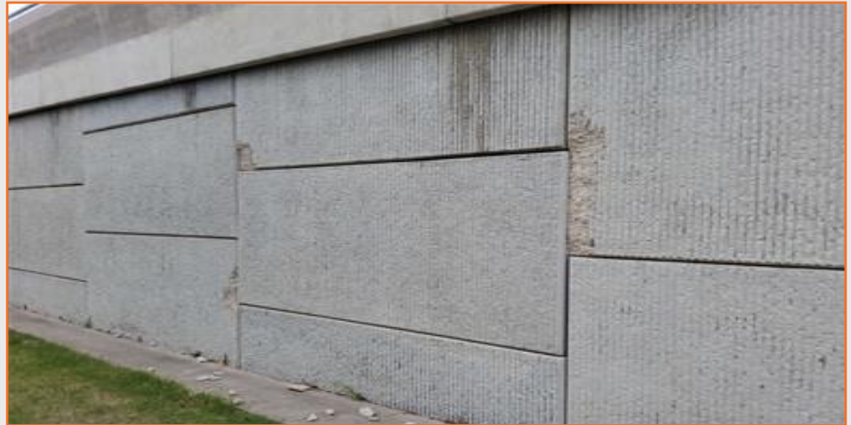
Figure 41: SRT retaining wall spalling SBFR at Ohio Dr.
