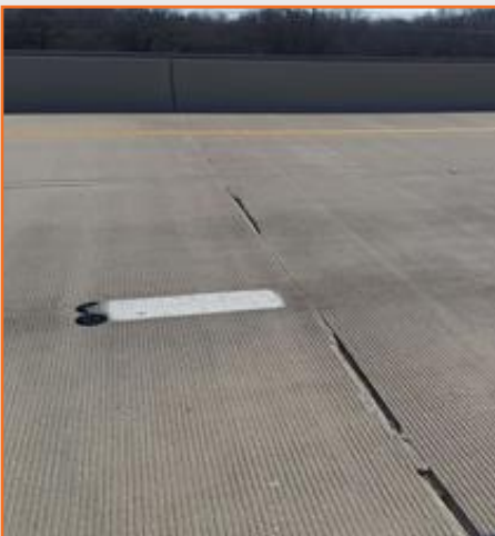
Figure 79: 360T bridge deck spalling SBML north of N Holland Rd.
