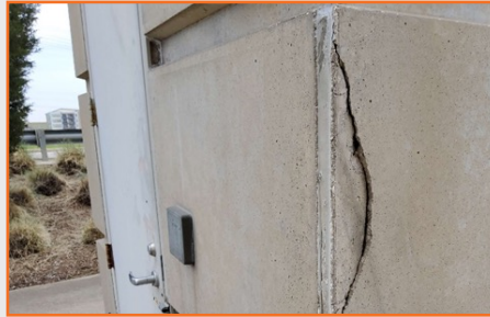
Figure 47: SRT MLG3 wall damage at IT building.
