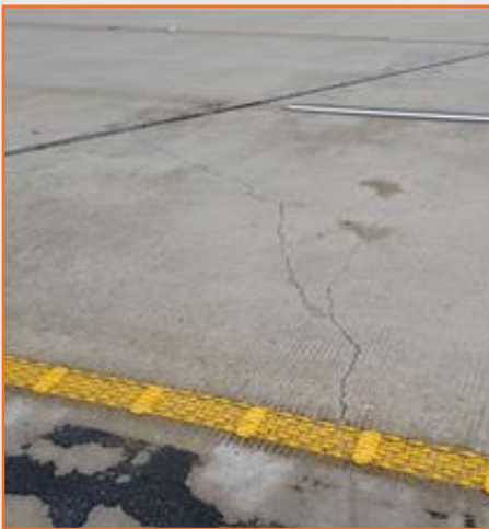
Figure 55: CTP approach slab cracking NBML south of Overton Ridge Blvd.
