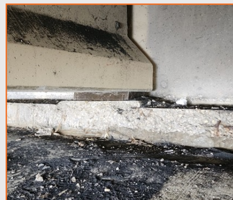
Figure 66: LLTB bridge abutment spalling with reinforcement exposed.
