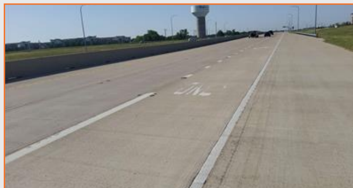
Figure 77: 360T pavement markings faded or missing SBML at Ragland Rd.
