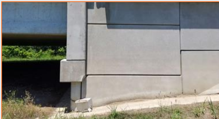
Figure 64: LLTB coping damage.
