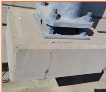
Figure 22: PGBT light pedestal cracking NBML just north of Pioneer Pkwy.
