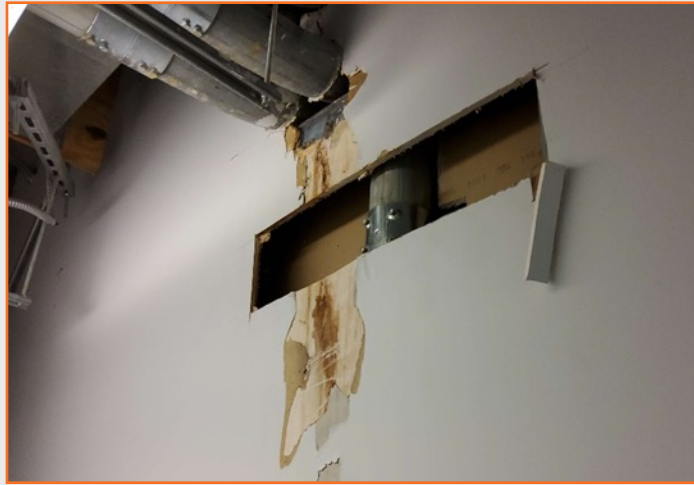
Figure 85: Frisco Operations Center gypsum board removed due to water infiltration at several locations.
