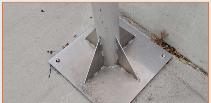
Figure 63: MCLB gantry camera stand missing bolts.
