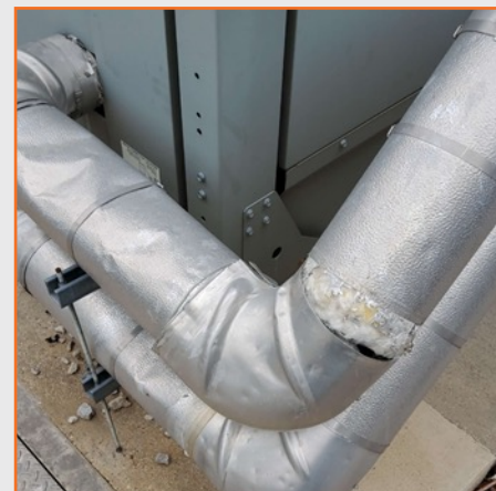
Figure 15: DNT MLP3 duct issues in mechanical yard.
