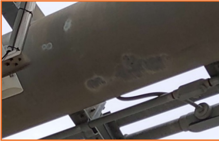
Figure 46: SRT MLG2 corrosion at gantry structure.
