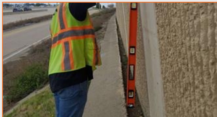
Figure 26: PGBT soundwall movement adjacent to NB exit ramp to Frankford Rd.
