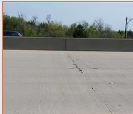
Figure 42: SRT bridge deck distress SBML north of S Lake Forest Dr.
