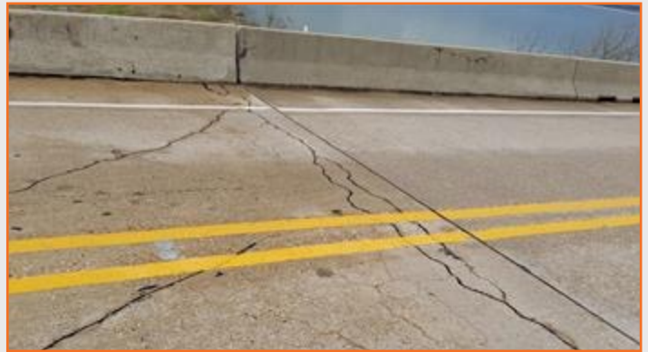
Figure 61: MCLB approach slab cracking.
