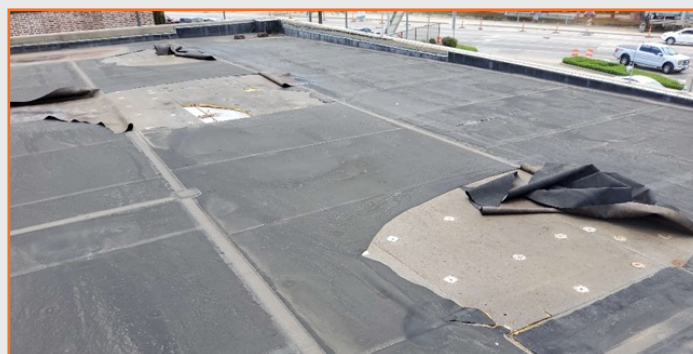
Figure 72: AATT roofing membrane damage.
