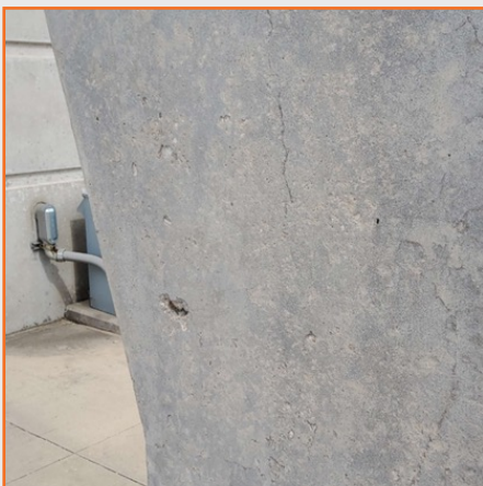
Figure 14: DNT MLG3 minor cracking and chipping at gantry columns.
