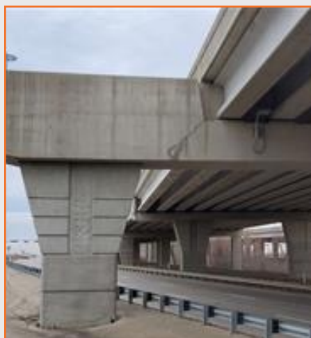
Figure 28: PGBT bridge bent cap cracking SBML south of S Forum Dr.
