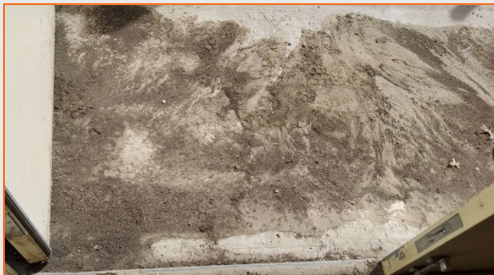
Figure 59: CTP Fiber Hut at IH-20 runoff entering building.
