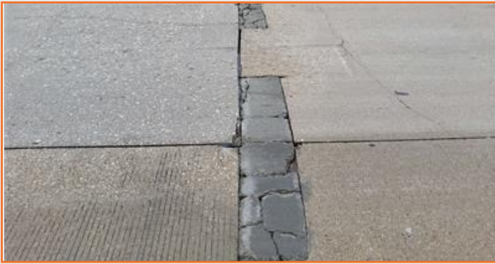
Figure 73: 360T concrete pavement distresses NBFR near Doryn Dr.
