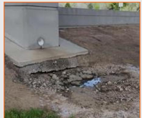
Figure 45: SRT bridge erosion SRT DC at US-75.
