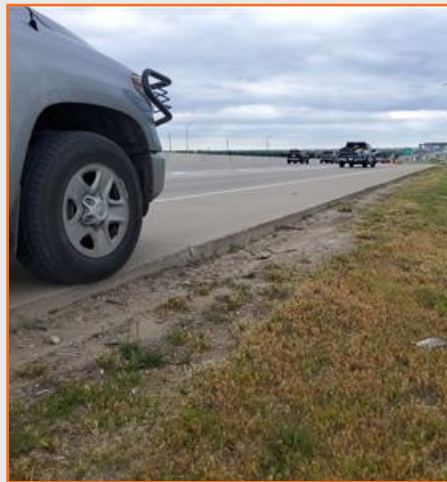
Figure 39: SRT pavement edge drop-off.
