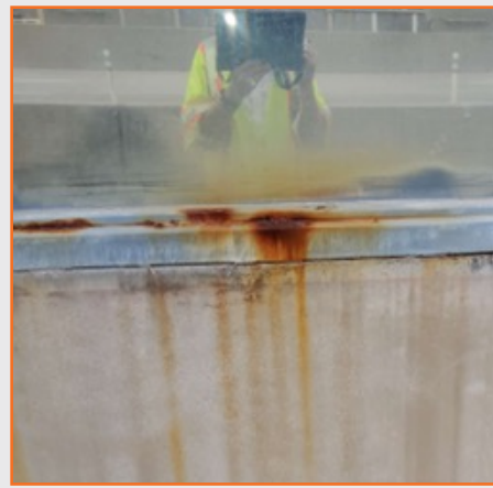
Figure 13: DNT MLG1 rust and paint repair at IT building.
