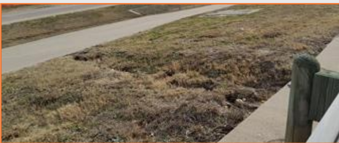
Figure 51: CTP embankment erosion NBML south of Sparks Dr.
