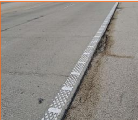
Figure 21: PGBT asphalt shoulder deterioration NBML just south of N. Garland Rd.
