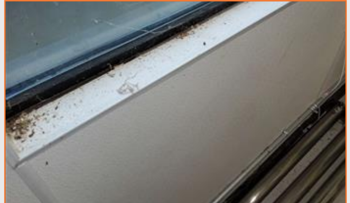
Figure 83: 360T Fiber Hut pest infestation.
