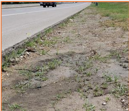
Figure 5: DNT pavement edge dropoff.
