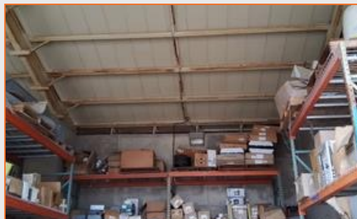
Figure 84: Plano Operations Center rust on steel frame of storage facility.
