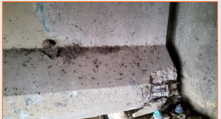
Figure 62: MCLB beam spalling with reinforcement exposed.
