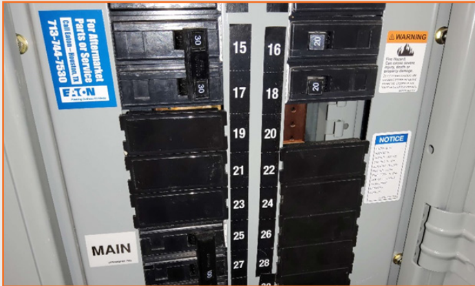
Figure 82: Panel board missing schedule.
