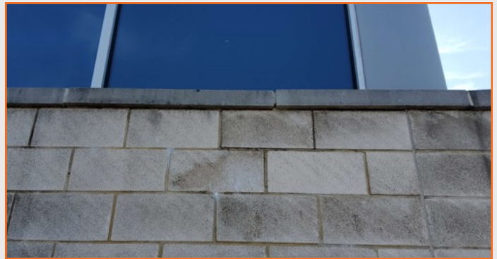
Figure 31: PGBT MLP7 masonry sealant and joint treatments past expected life-cycle.
