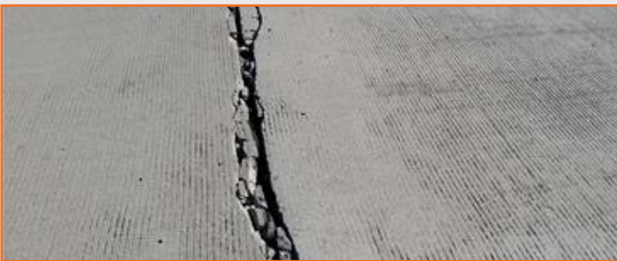
Figure 49: CTP concrete pavement joint deterioration SBML north of Arborlawn Dr.
