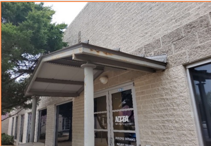
Figure 86: Gleneagles Office Complex ferrous metal coating failure.
