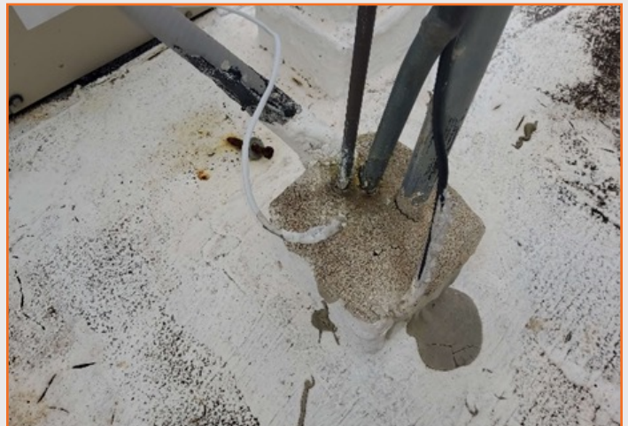
Figure 87: Gleneagles Office Complex roof deterioration.
