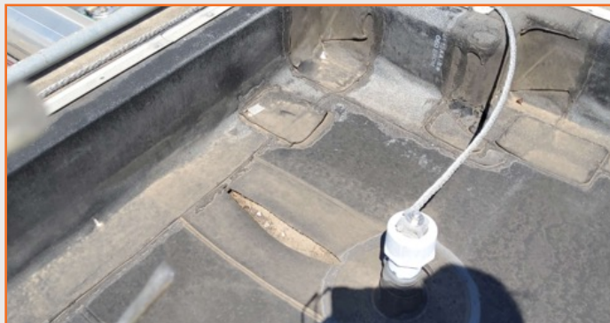
Figure 32: PGBT MLG6 gantry roof deterioration.
