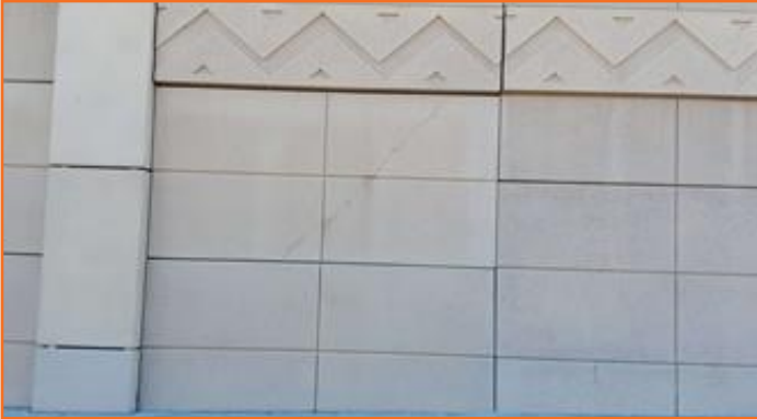
Figure 53: CTP MSE retaining wall panel cracking NBML north of Southwest Blvd.
