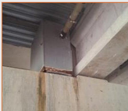
Figure 67: LLTB rusted utility box on bent cap.
