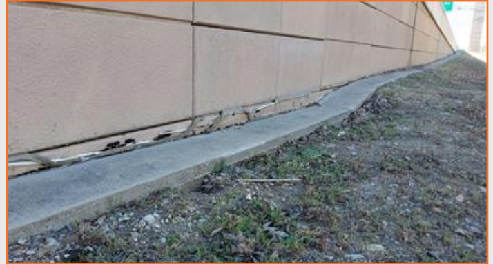
Figure 54: CTP MSE racked panels and wall mow strip settlement SBML adjacent to UPRR Rail Yard.
