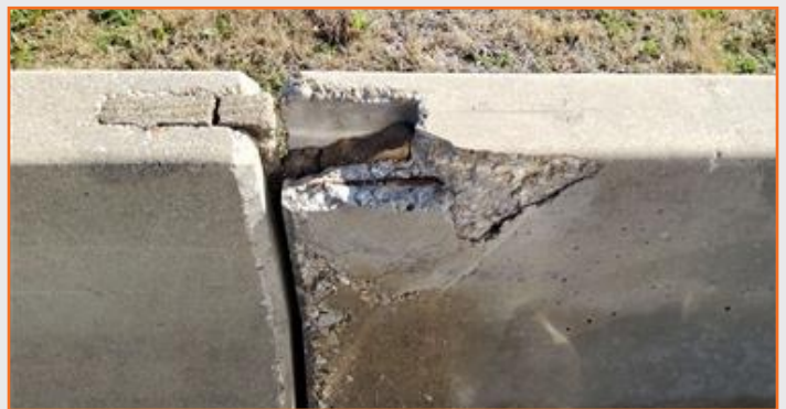
Figure 74: 360T concrete barrier damage with reinforcement exposed SBML south of SE Green Oaks Blvd.
