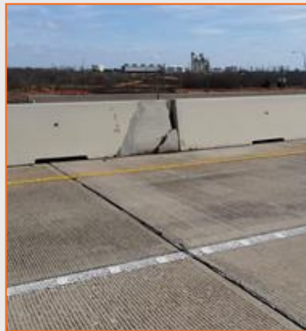
Figure 56: CTP bridge rail spalling SBML at Sparks Dr.
