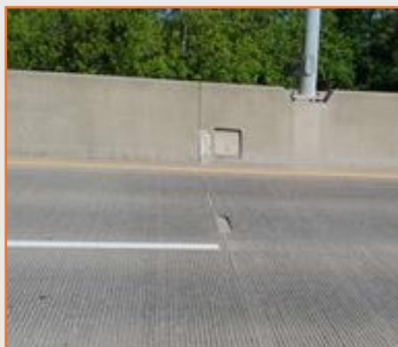
Figure 65: LLTB bridge deck spalling EBML.
