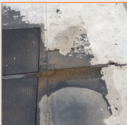
Figure 16: DNT MLP4 roof deterioration.
