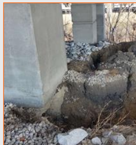
Figure 29: PGBT under bridge erosion SBML south of S Forum Dr.
