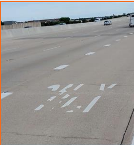
Figure 38: SRT pavement markings faded or missing NBML south of W Hebron Pkwy.
