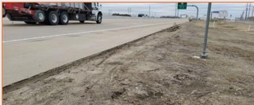
Figure 24: PGBT pavement edge drop-off.
