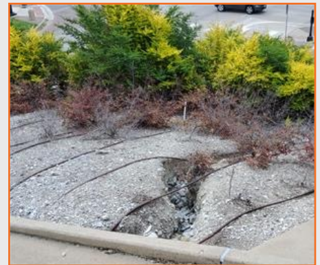
Figure 4: DNT erosion SBML S. of Gaylord Pkwy.
