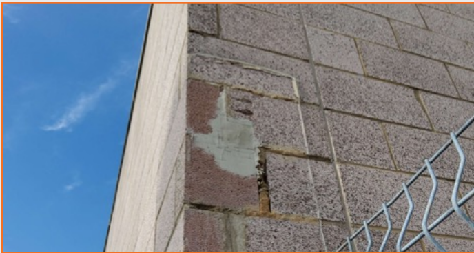
Figure 30: PGBT MLP7 deteriorated masonry joints.
