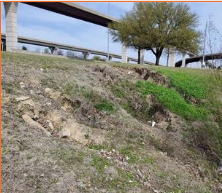
Figure 18: PGBT roadside erosion adjacent to SBML at IH-30 in Garland.
