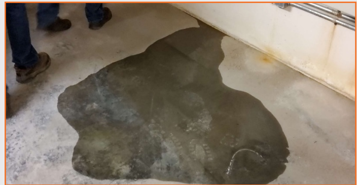
Figure 33: PGBT MLP6 tunnel leaks.
