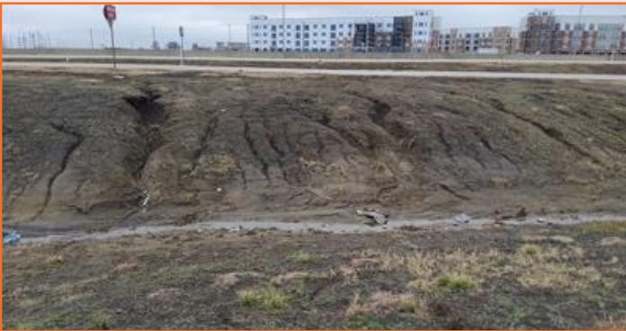
Figure 75: 360T embankment erosion between NB mainlanes and frontage road near Heritage Pkwy.
