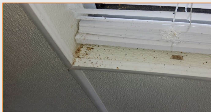
Figure 34: PGBT MLG12 pest control at Fiber Hut.
