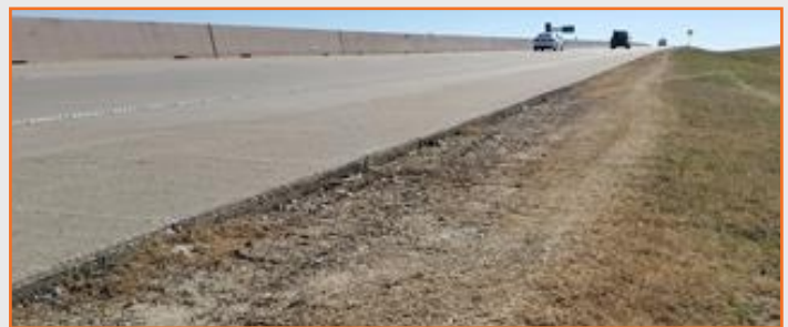
Figure 52: CTP pavement edge drop-off.
