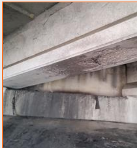
Figure 80: 360T bridge beam and concrete riprap spalling at SE Green Oaks Blvd.
