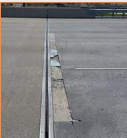
Figure 27: PGBT bridge deck spalling EBML at DNT.
