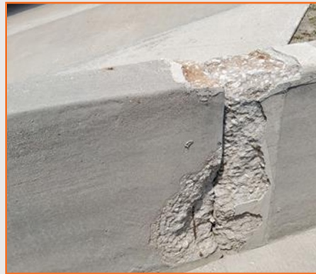
Figure 3: DNT concrete rail damage SBML south of Eldorado Pkwy.
