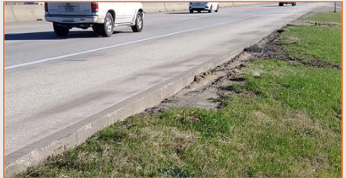
Figure 76: 360T pavement edge drop-off.
