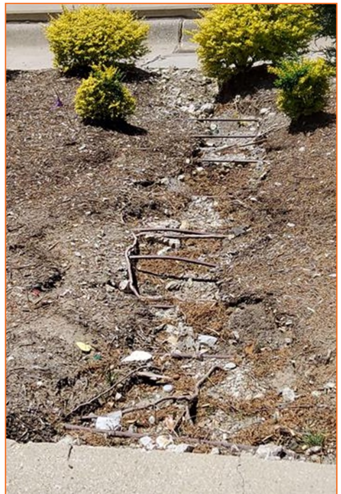
Figure 3: DNT erosion SBML S. of Gaylord Pkwy.
