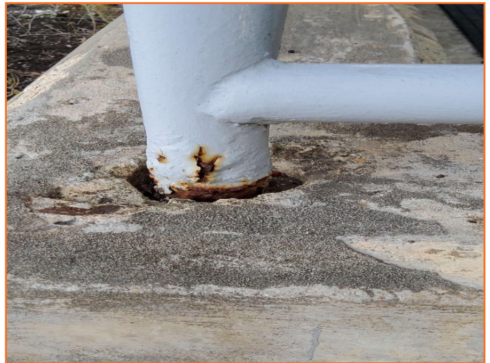
Figure 59: Gleneagles 5900 – handrail rusting at base
