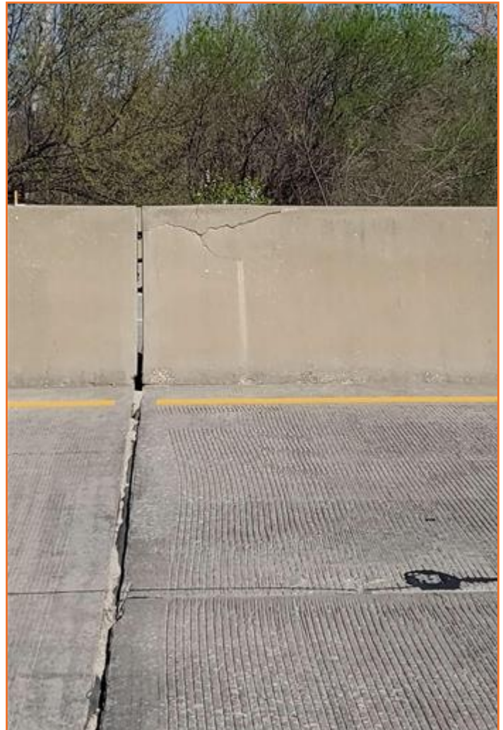
Figure 44: LLTB pavement seal missing/damaged
