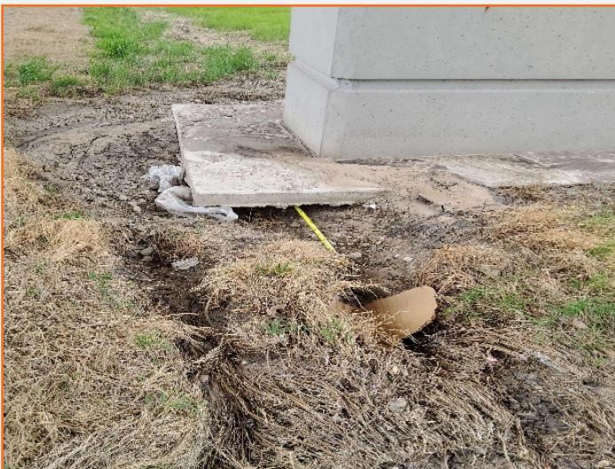
Figure 27: SRT erosion NB-US75-NB SRT DC
