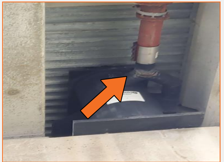
Figure 48: LLTB AquaShield pipe welding broken
