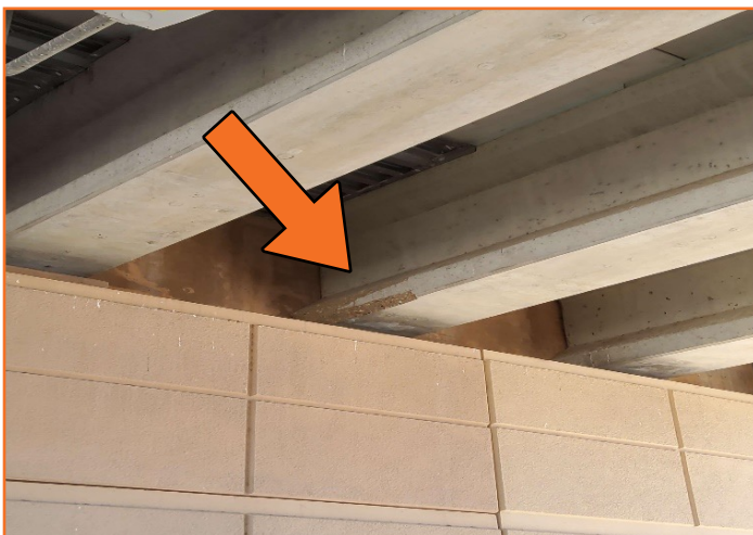
Figure 37: CTP bridge beam spall at Edwards Ranch Rd.
