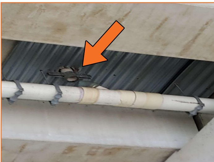
Figure 22: PGBT at Lake Ray Hubbard Deck drain pipe disconnected NB bent No. 21
