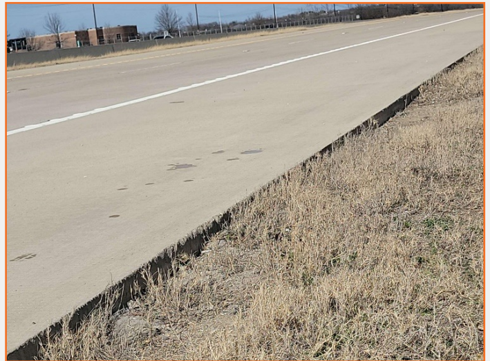
Figure 52: 360T pavement edge drop-off North of Ragland Rd.
