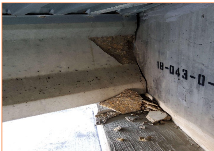
Figure 30: SRT beam end spall SB structure at Hardin Blvd.
