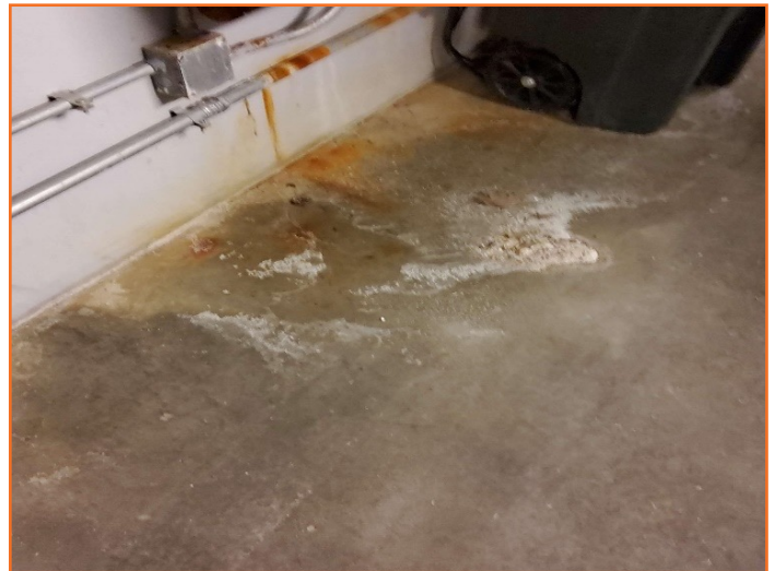
Figure 23: PGBT MLP 7 – rust staining on floor
