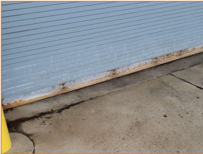
Figure 56: Ohio – rust on overhead door seals
