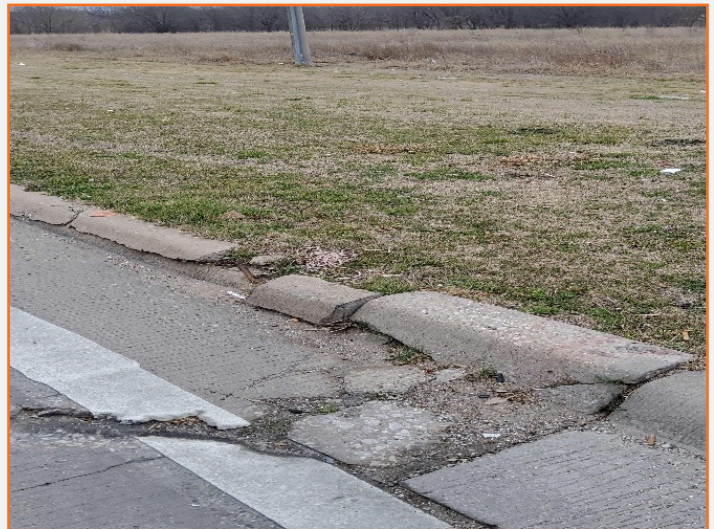
Figure 28: SRT curb damage NBR at Razor Blvd.
