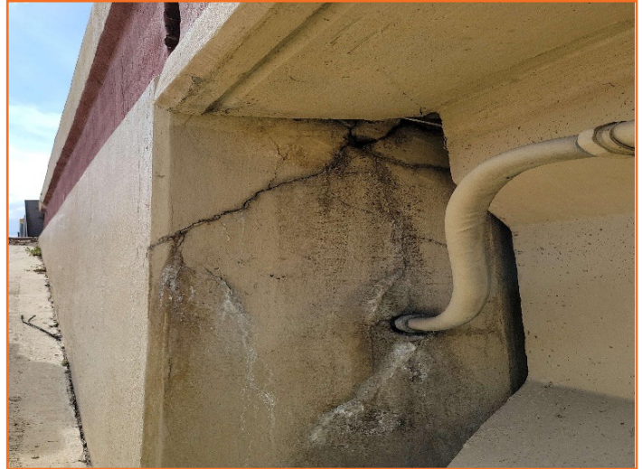
Figure 19: PGBT backwall cracking/spalling on SB structure at E. Rosemeade Pkwy.
