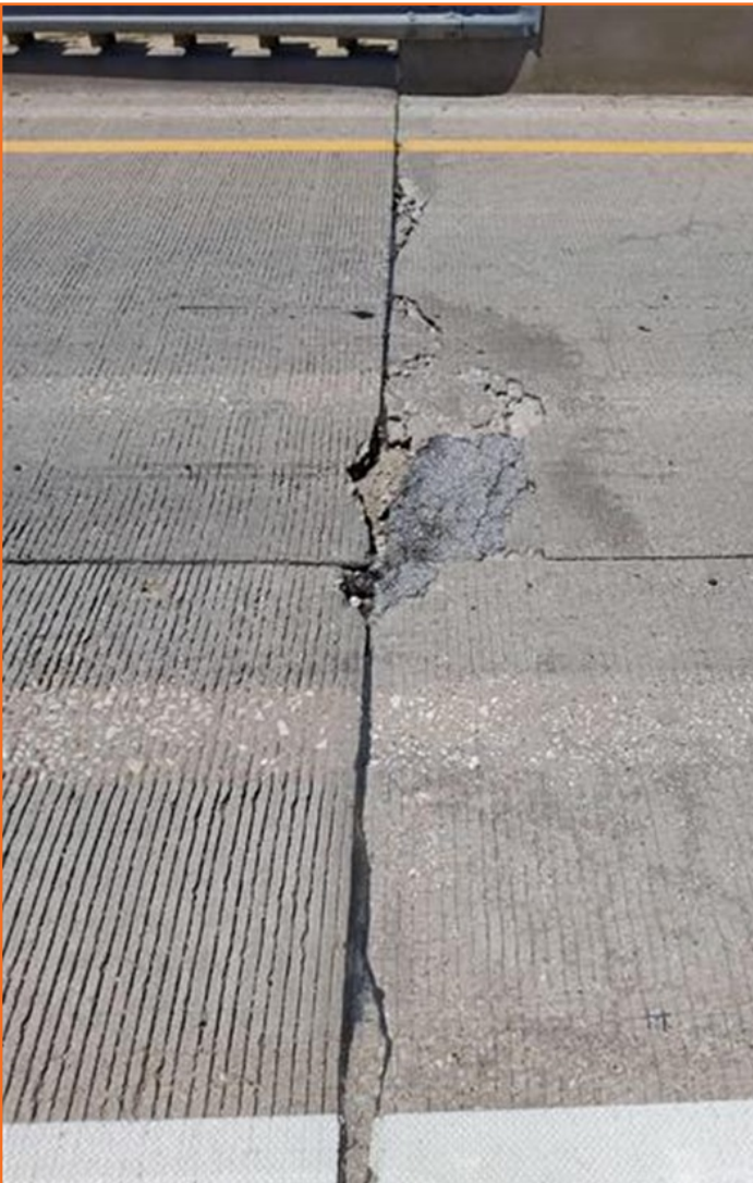
Figure 5: DNT pavement joint deterioration NBML N. of Eldorado Pkwy.
