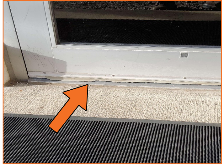
Figure 58: Gleneagles 5900 – door sweeps deteriorated
