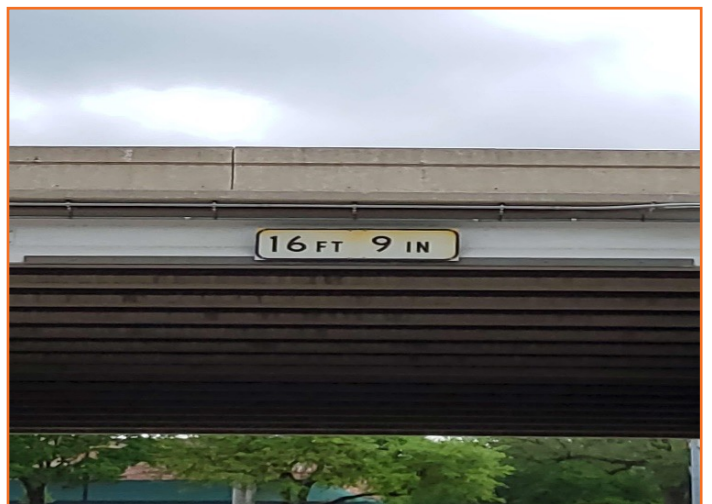
Figure 8: DNT clearance sign faded SB U-Turn at Trinity Mills Rd.
