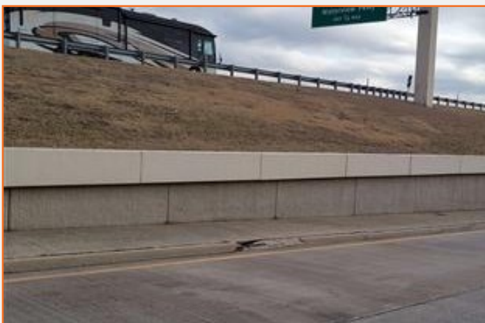
Figure 14: PGBT curb damage NBRF at Conflans Rd.
