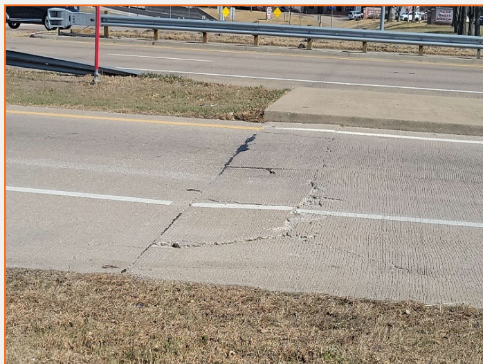
Figure 17: PGBT pavement cracking SB exit ramp to Hwy. 78
