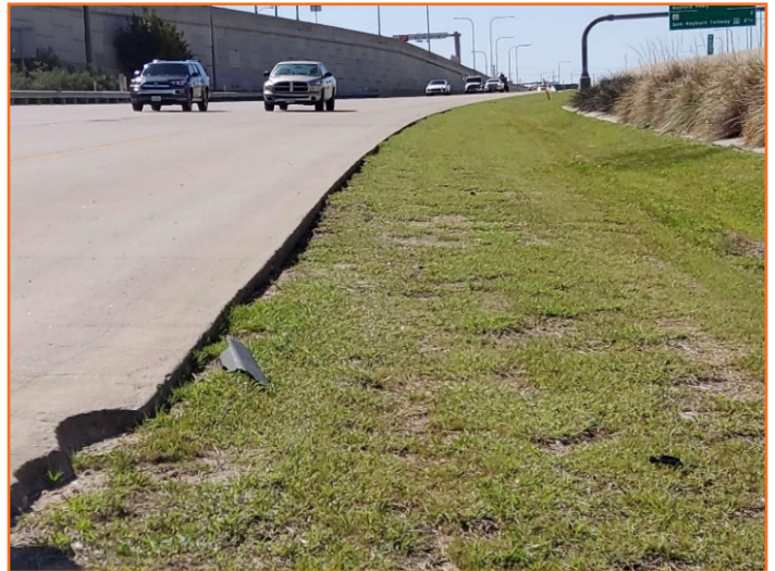
Figure 6: DNT pavement edge drop-off NBML S. of Stonebrook Pkwy.
