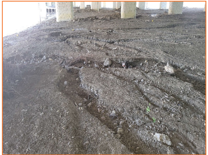
Figure 20: PGBT erosion under bridge SBFR South of N. Carrier Pkwy.
