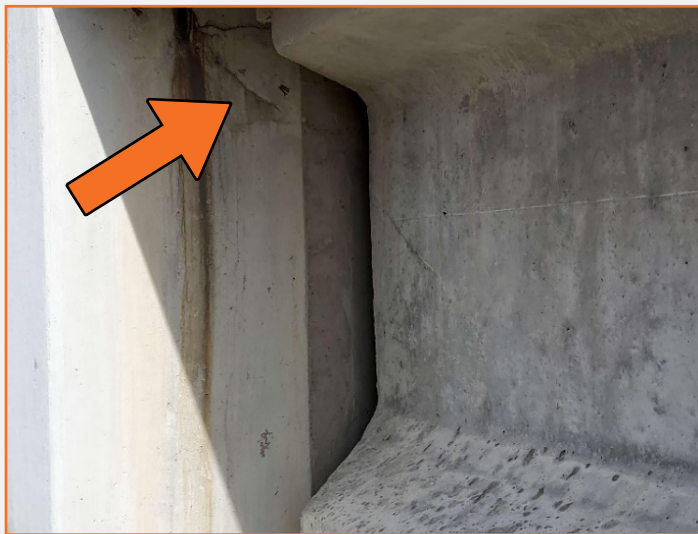
Figure 54: 360T backwall cracking at Bowman Branch bridge
