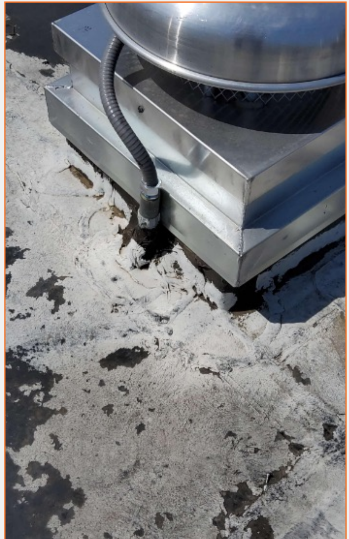
Figure 13: DNT MLP4 – deteriorated roof
