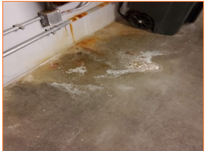
Figure 23: PGBT MLP 7 – rust staining on floor
