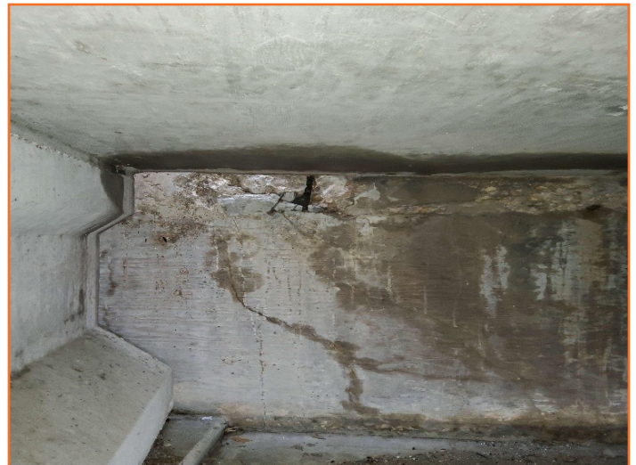
Figure 11: DNT bridge abutment cracking NB at Harvest Hill Rd.
