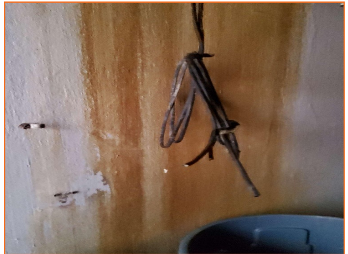
Figure 24: PGBT MLP 8 – rust developing on wall
