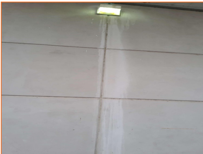
Figure 57: Frisco – staining at light fixture
