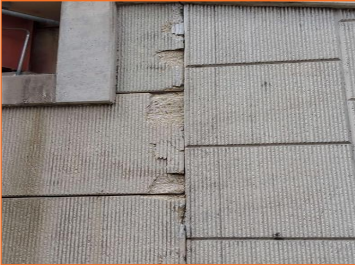
Figure 18: PGBT retaining wall panel spalling SB at N. MacArthur Blvd.
