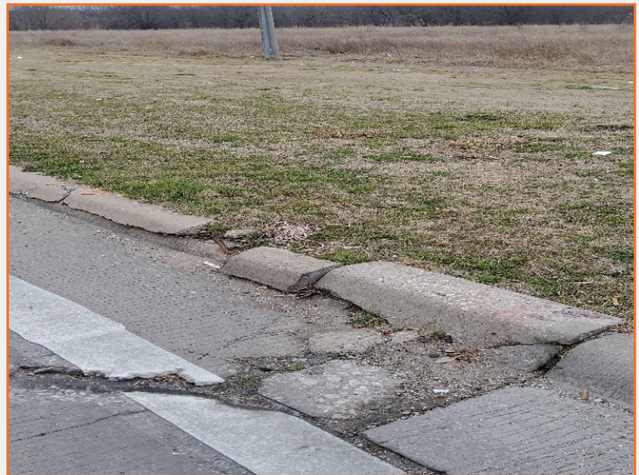
Figure 28: SRT curb damage NBR at Razor Blvd.
