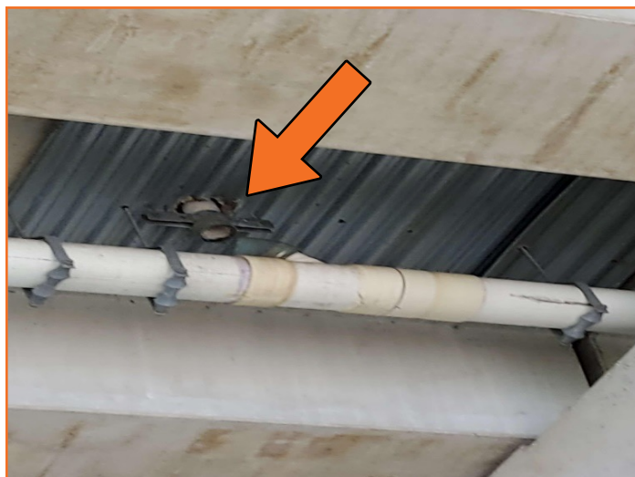
Figure 22: PGBT at Lake Ray Hubbard Deck drain pipe disconnected NB bent No. 21
