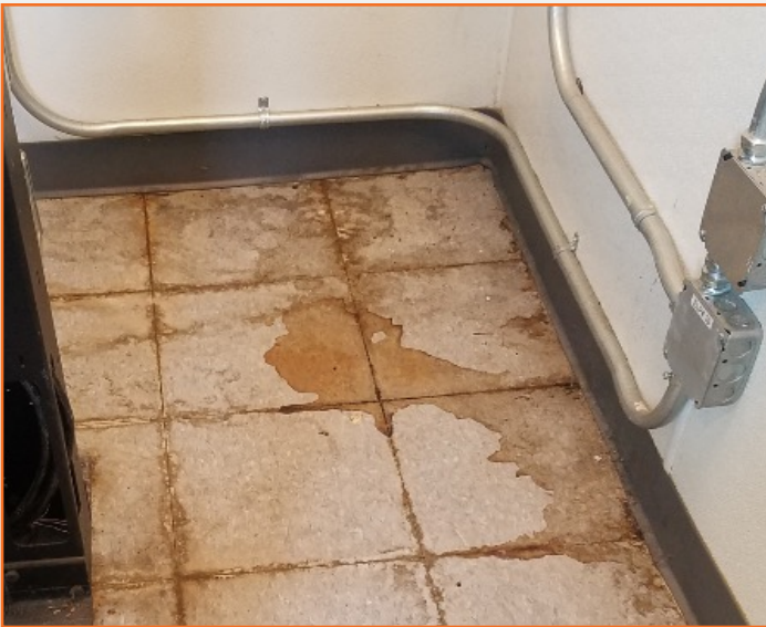
Figure 12: DNT MLP3 – floor damage from water intrusion
