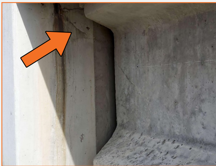
Figure 54: 360T backwall cracking at Bowman Branch bridge
