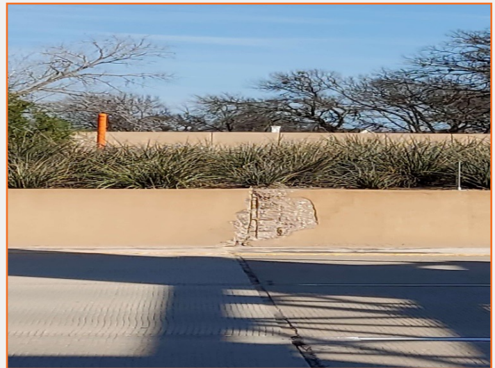
Figure 36: CTP barrier spalling NB just South of Arborlawn Dr.
