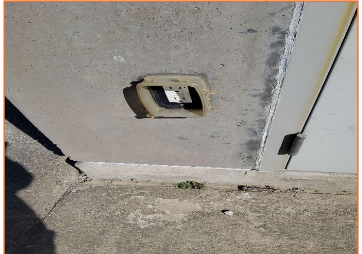
Figure 31: SRT MLG 2 – electrical box cover missing
