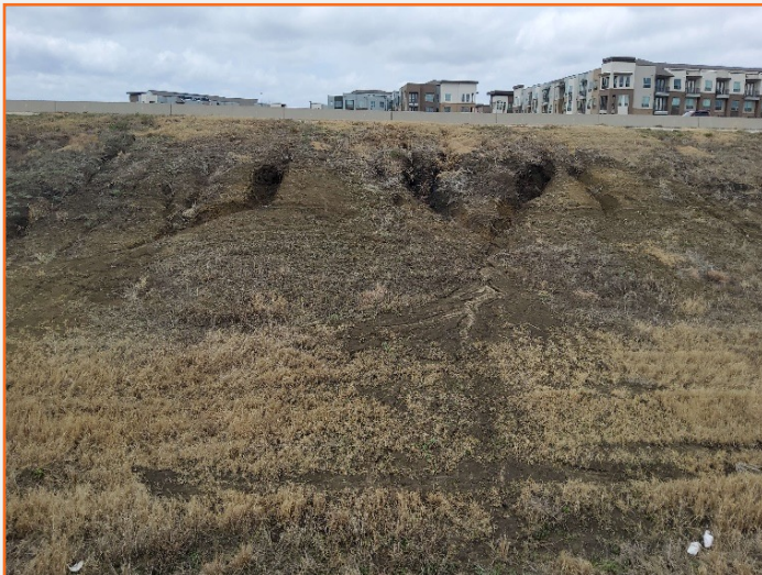
Figure 51: 360T embankment erosion NB North of Heritage Pkwy.
