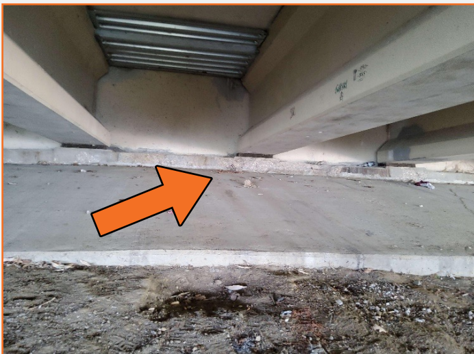
Figure 47: LLTB abutment spalling at East end of bridge
