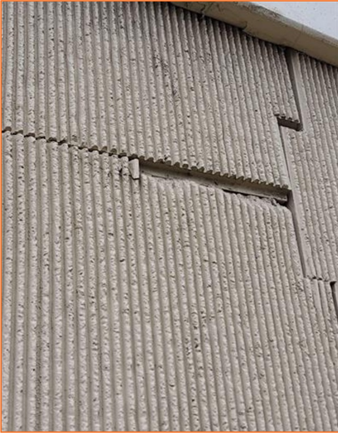
Figure 9: DNT retaining wall panel crack NBML S. of IH-635
