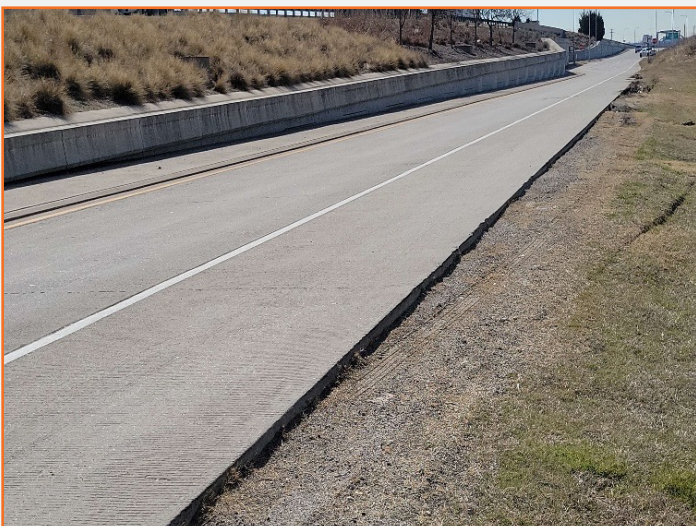
Figure 16: PGBT pavement edge drop-off SB exit ramp to Merritt Rd.
