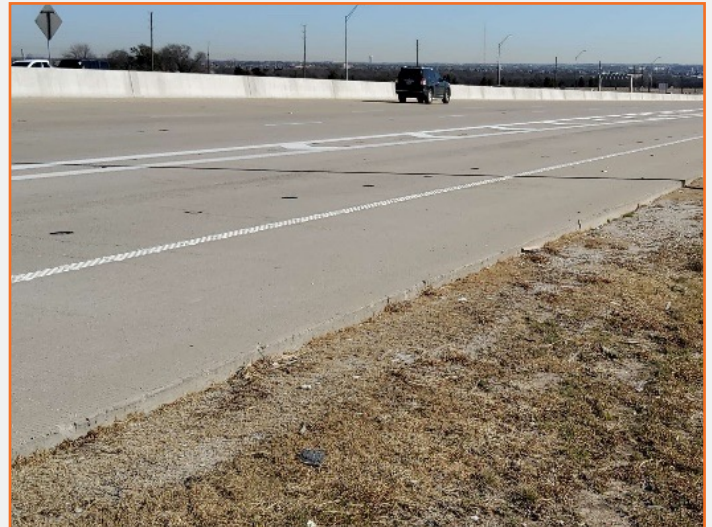
Figure 26: SRT pavement edge drop-off NB exit ramp to Independence Pkwy.
