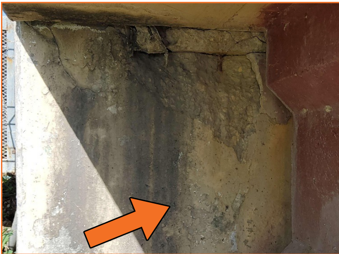
Figure 43: MCLB backwall spalling at West abutment
