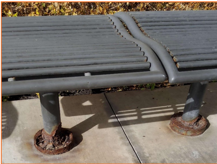
Figure 60: Gleneagles 5910 – bench bases rusting
