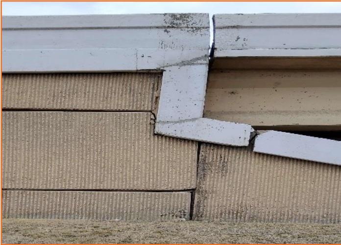
Figure 29: SRT misaligned wall panel at NB 121 Bus. DC
