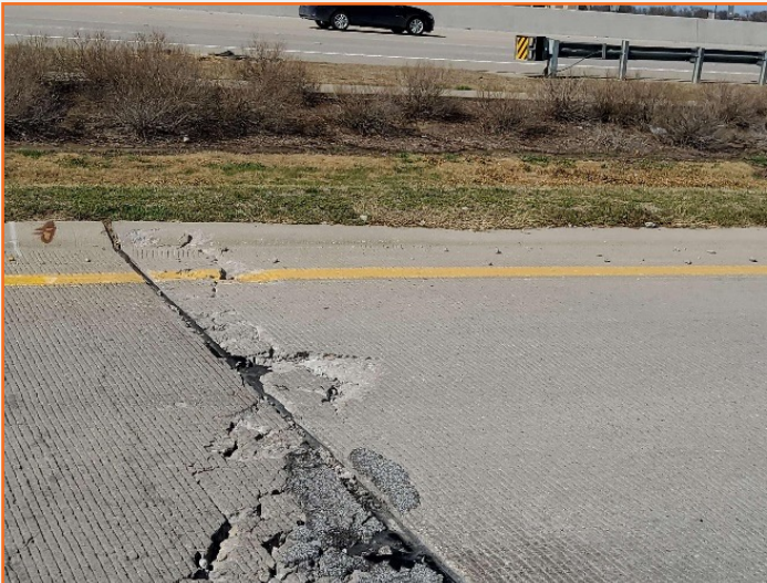
Figure 25: SRT pavement cracking/spalling NB exit ramp to N. Josey Ln.
