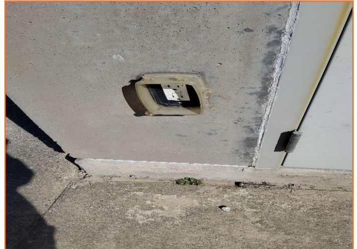
Figure 31: SRT MLG 2 – electrical box cover missing
