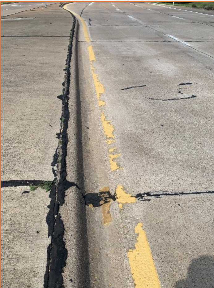
Figure 40: MCLB faded or missing pavement markings
