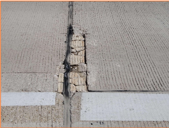
Figure 4: DNT pavement distress SBML N. of Windhaven Pkwy.
