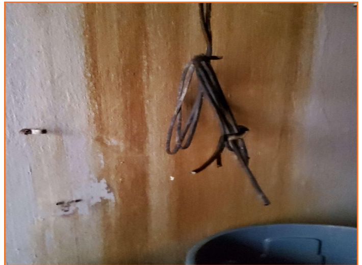
Figure 24: PGBT MLP 8 – rust developing on wall
