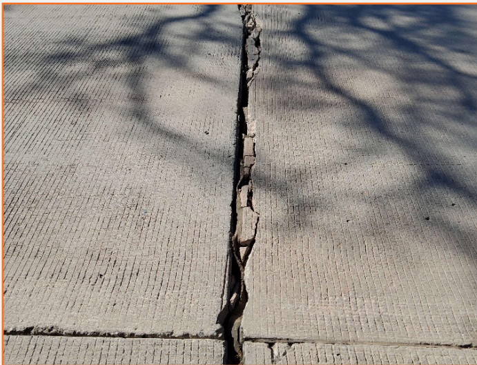
Figure 35: CTP pavement joint deterioration at SB exit ramp to Arborlawn Dr.
