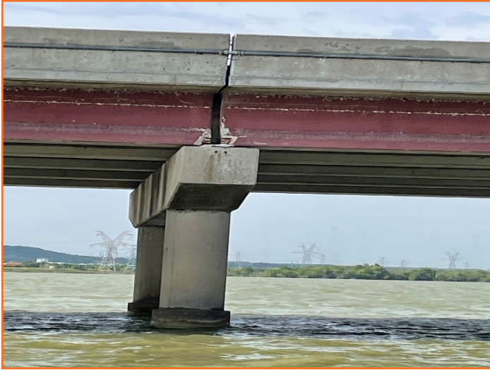
Figure 42: MCLB typical beam end spall
