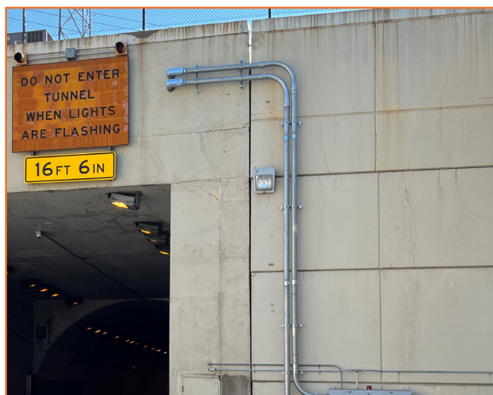
Figure 50: AATT cracked and spalled wall panels on West end tunnel entrance
