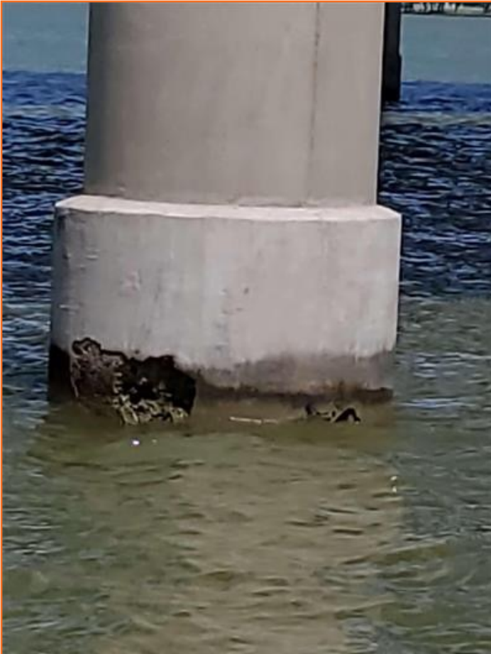
Figure 21: PGBT at Lake Ray Hubbard column spall NB bent No. 48
