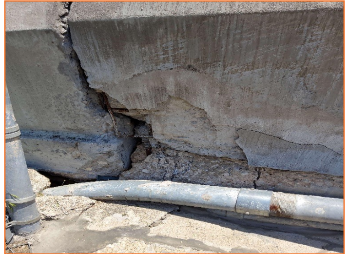
Figure 10: DNT concrete rail damage SB at Maple Ave.
