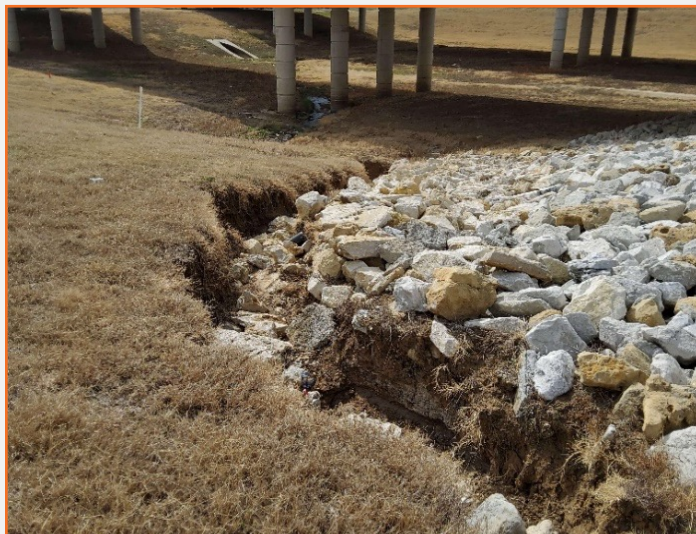
Figure 55: 360T erosion around riprap at Walnut Creek bridge
