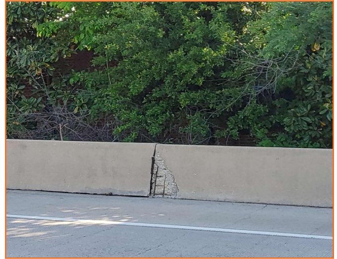
Figure 2: DNT barrier wall spall NBML S. of Knight St.
