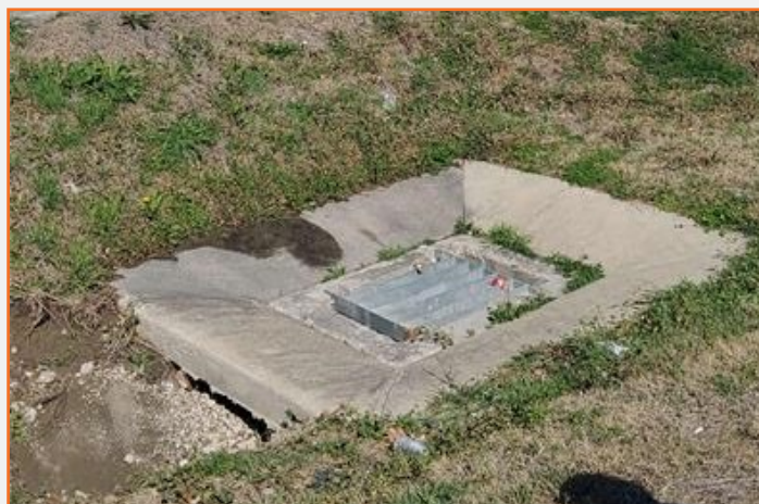
Figure 15: PGBT erosion under inlet NBRF North of W. Pioneer Pkwy.
