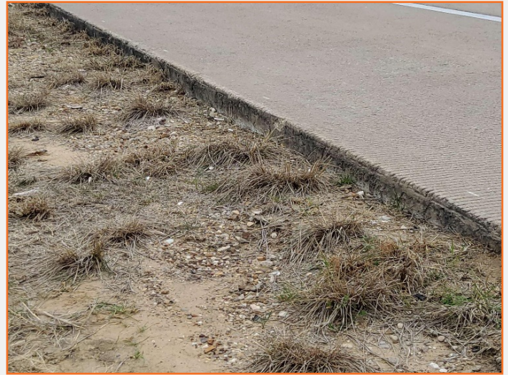
Figure 34: CTP pavement edge drop-off NB just South of FM 917
