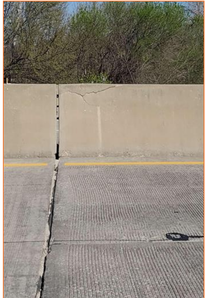
Figure 44: LLTB pavement seal missing/damaged
