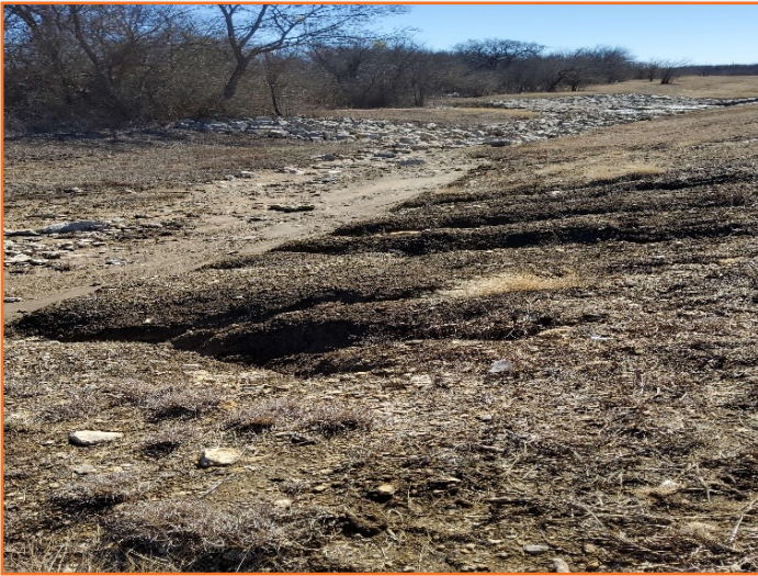
Figure 33: CTP embankment erosion – NB North of CR 1015
