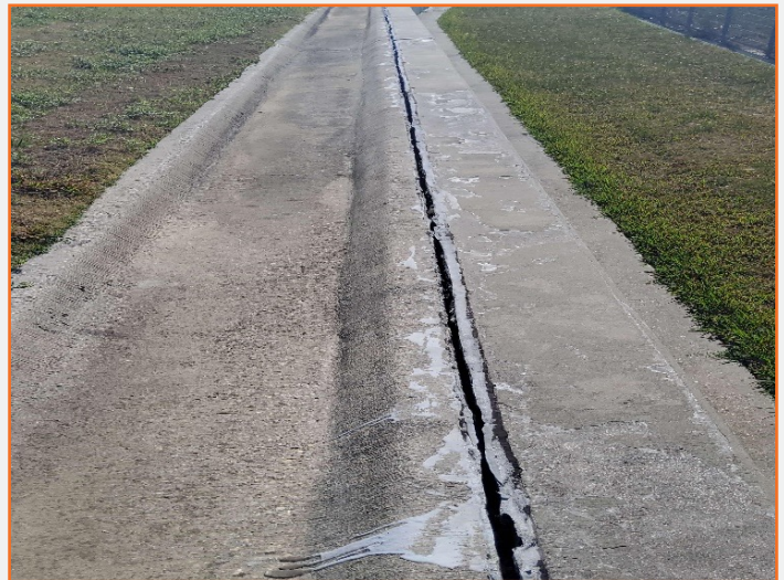
Figure 41: MCLB flume unsealed at wall East end of bridge
