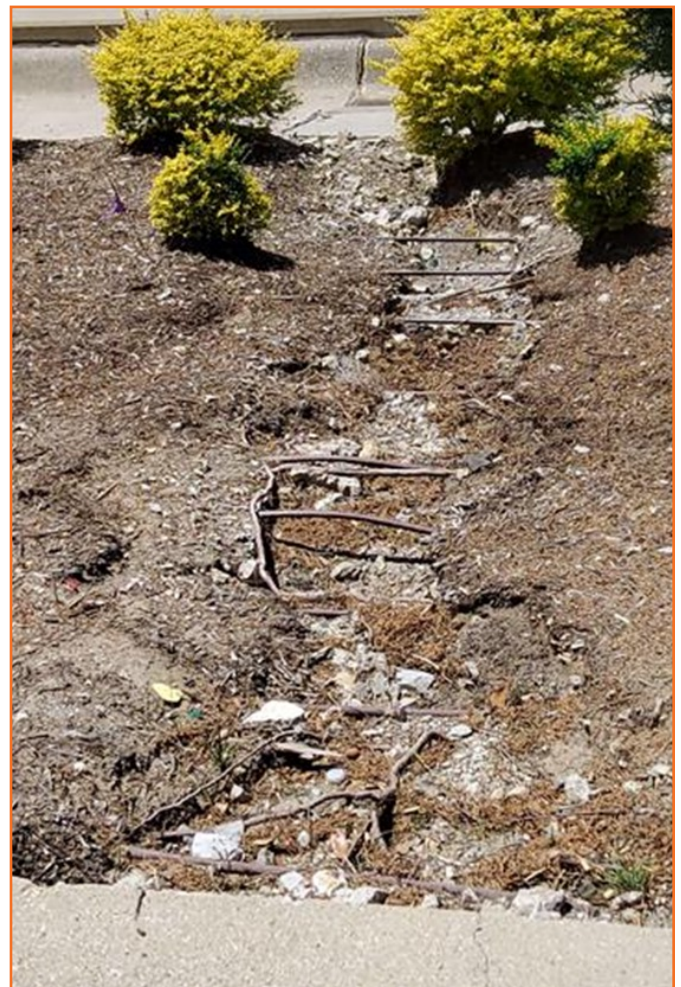
Figure 3: DNT erosion SBML S. of Gaylord Pkwy.
